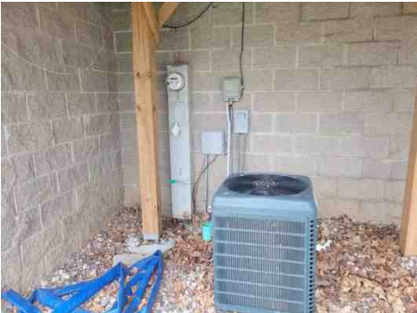
AC / Electrical Meter
