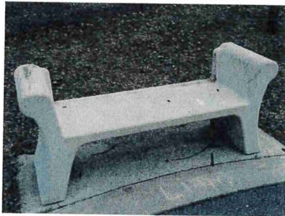
Back support on bench is missing
