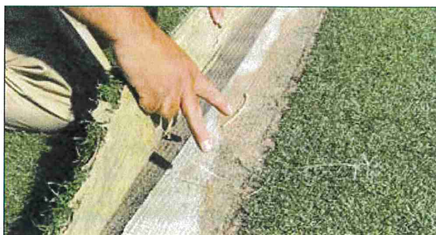
Major repairs required - call AstroTurf for help
