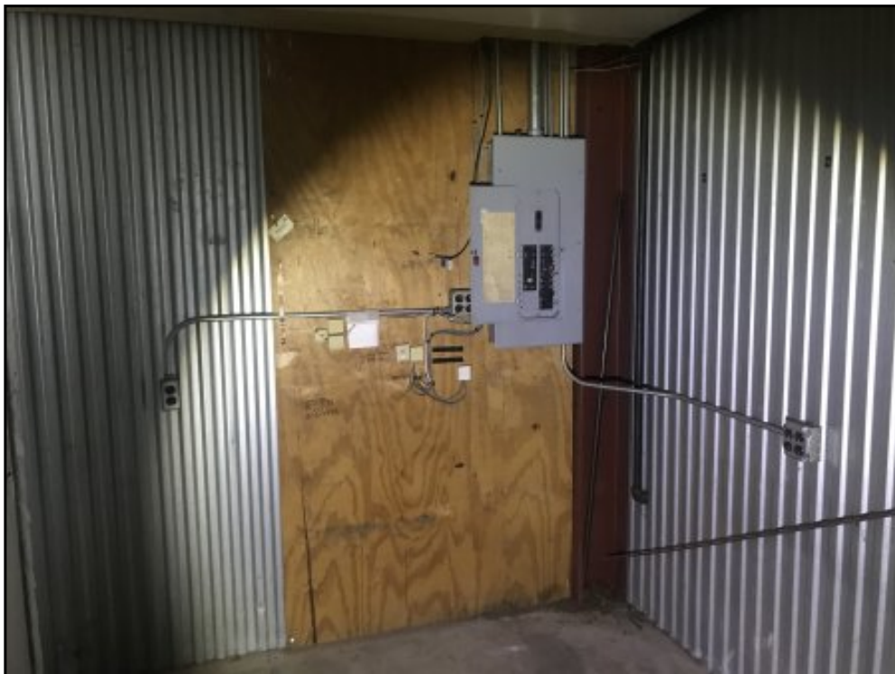
Electrical panel inside building
