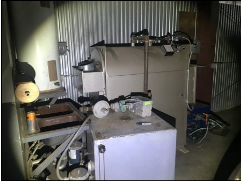
Hot water heater and furnace
