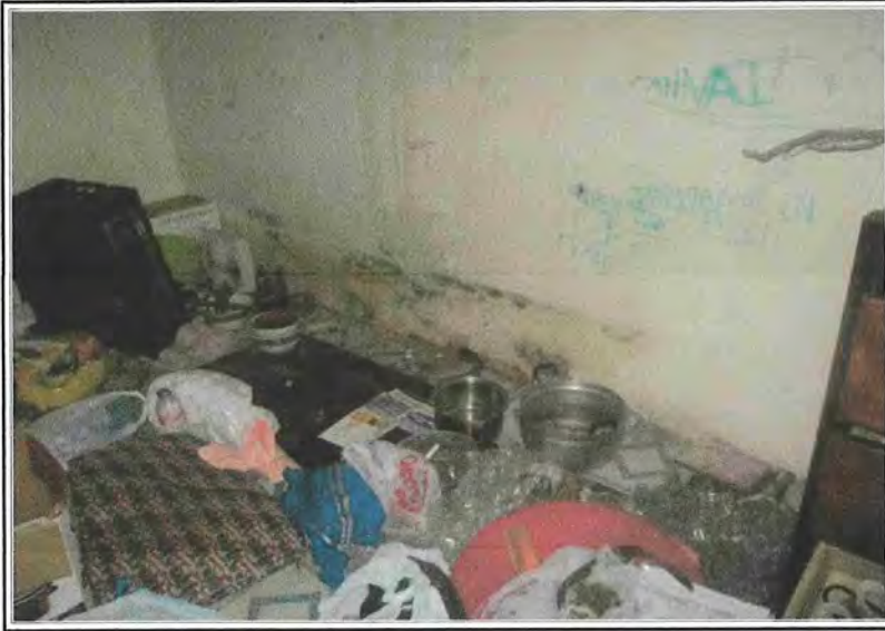
BEDROOM WALL MOLD
