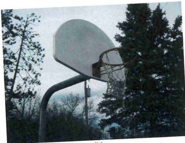
Basketball net in poor condition
