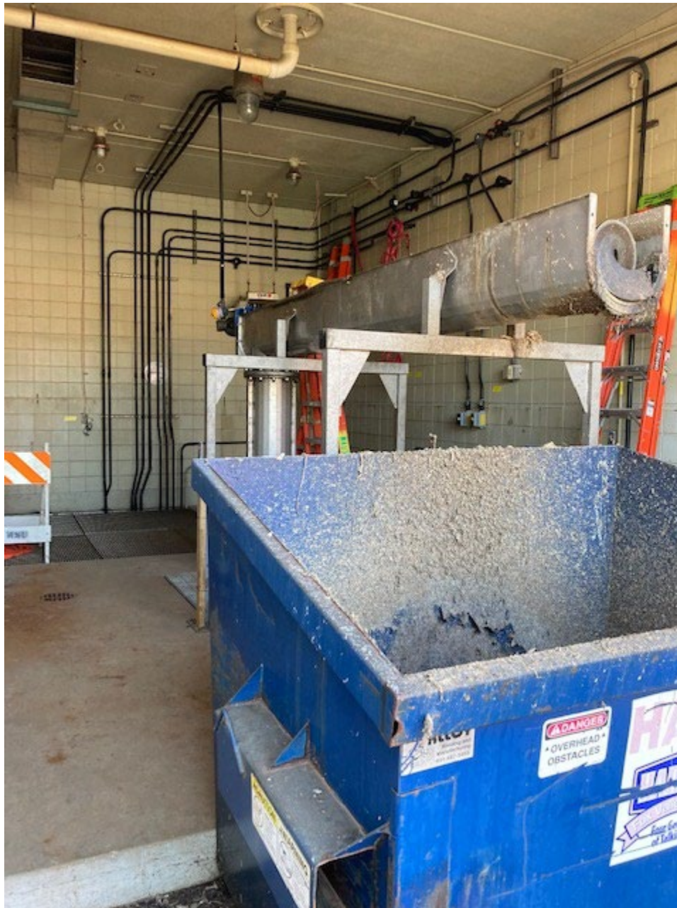
Screw Conveyor – Horizontal at-grade section
