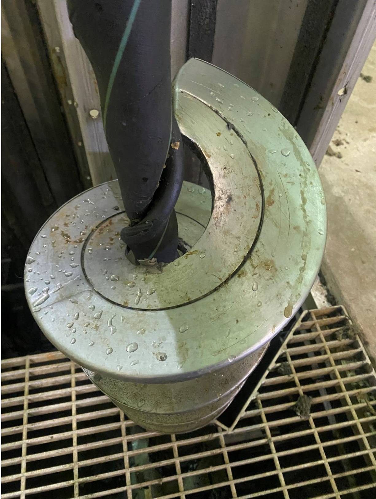
Torque twisted the shaft and this needed to be rebuilt along with gear box
