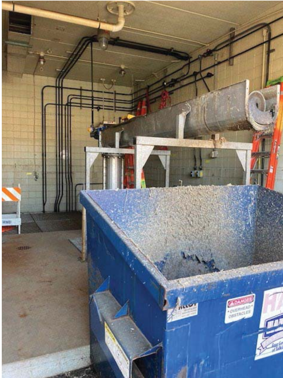
Screw Conveyor – Horizontal at-grade section
