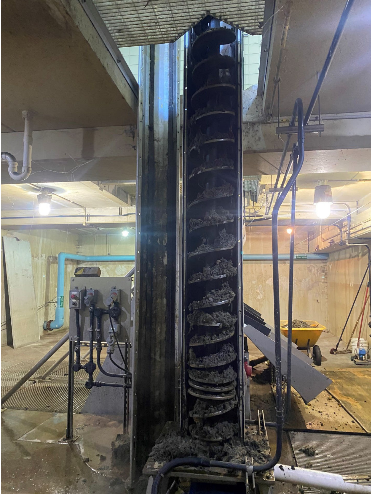
Vertical Screw Conveyor – Below grade vertical shaft open clogged too much weight for gear box
