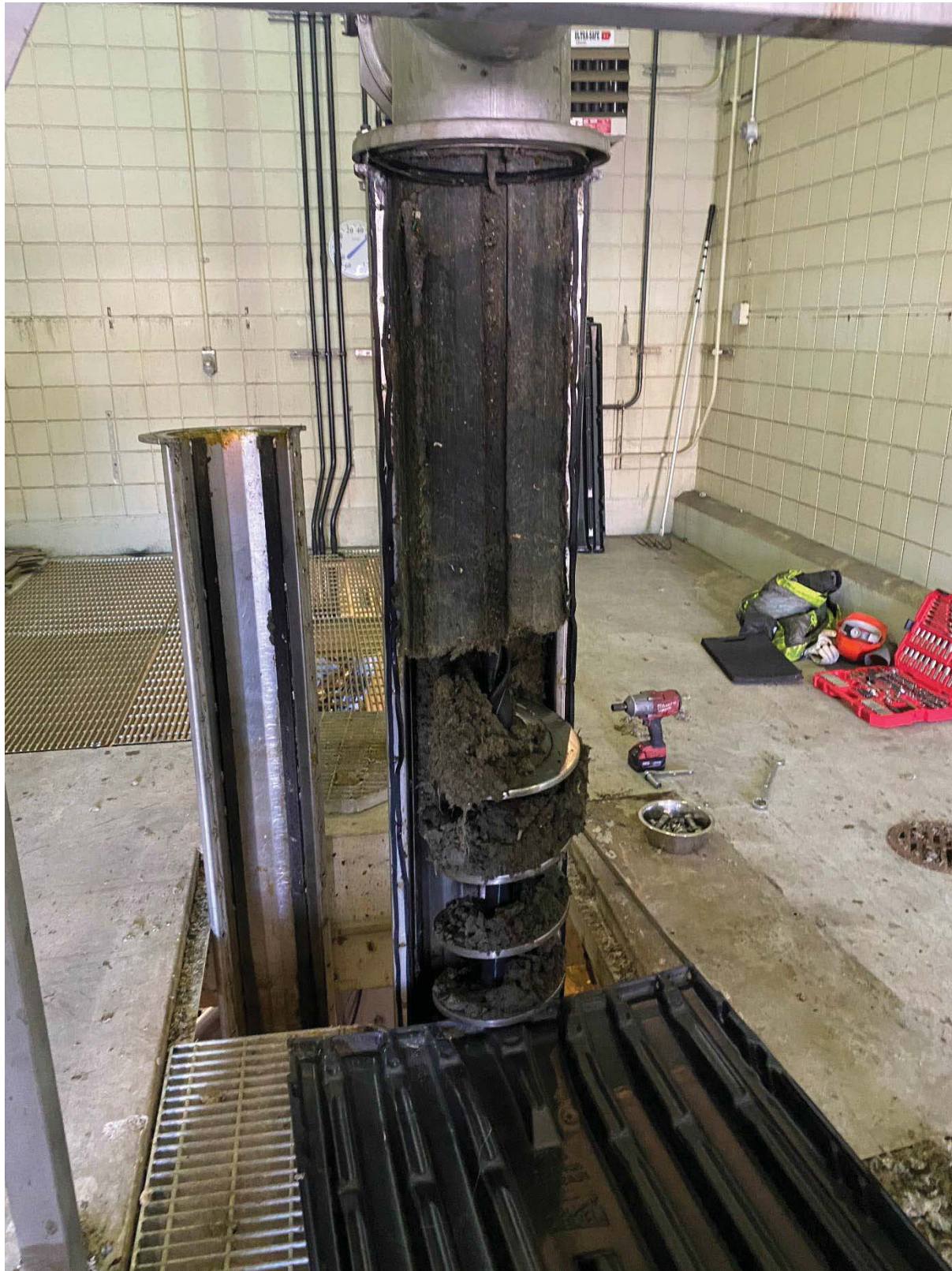
Screw conveyor at grade opened was clogged with debris, transition to horizontal screw
