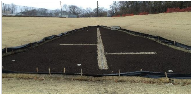
UAZ: 3,500-square-foot west bioretention basin serving low flows from 19-acre watershed with pretreatment and upflow level spreader.
