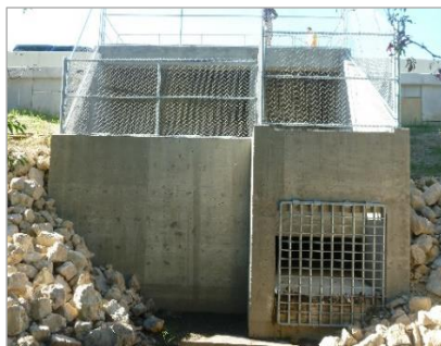
Hydrodynamic separator (coanda screen) pretreatment device treating Beltline flows prior to discharge to Curtis Pond.
