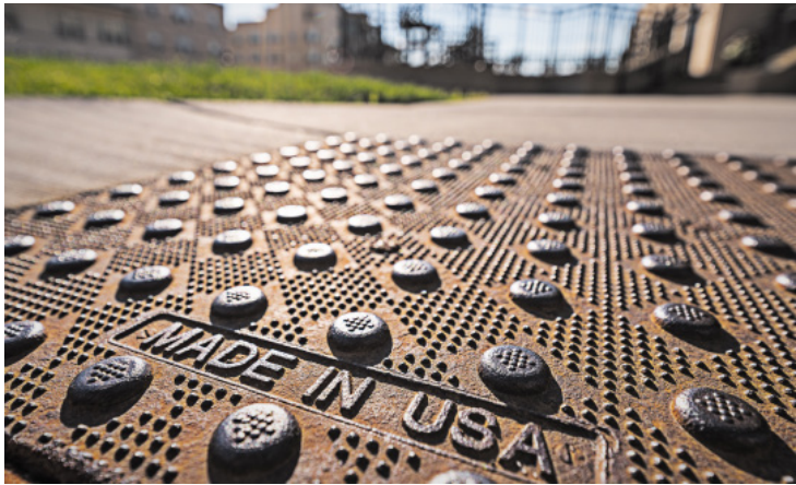
Detectable Warning Plates located between pedestrian areas and parking to meet ADA (cast iron with weathered natural patina)
