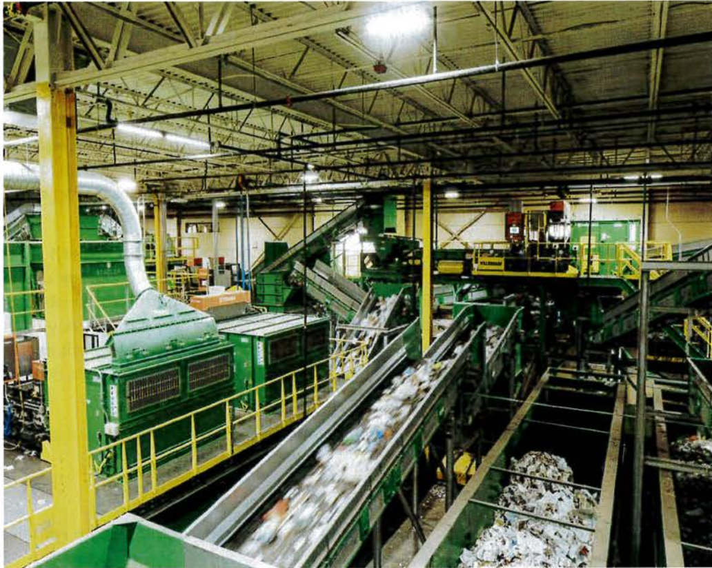
State-of-the-art Sorting Technology at work in the WM Germantown Recycling Facility
