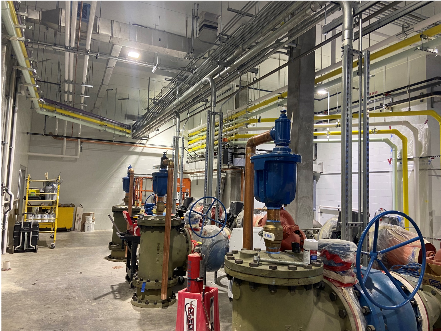
Process Bldg. – High Service Pump Area with Chemical Piping
