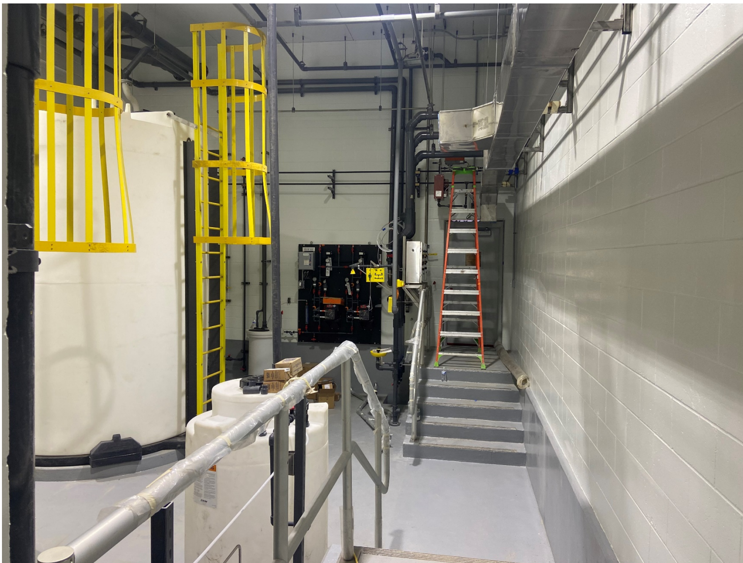
Process Bldg. – Chemical Storage Room with Fill Instrumentation Panels Installed
