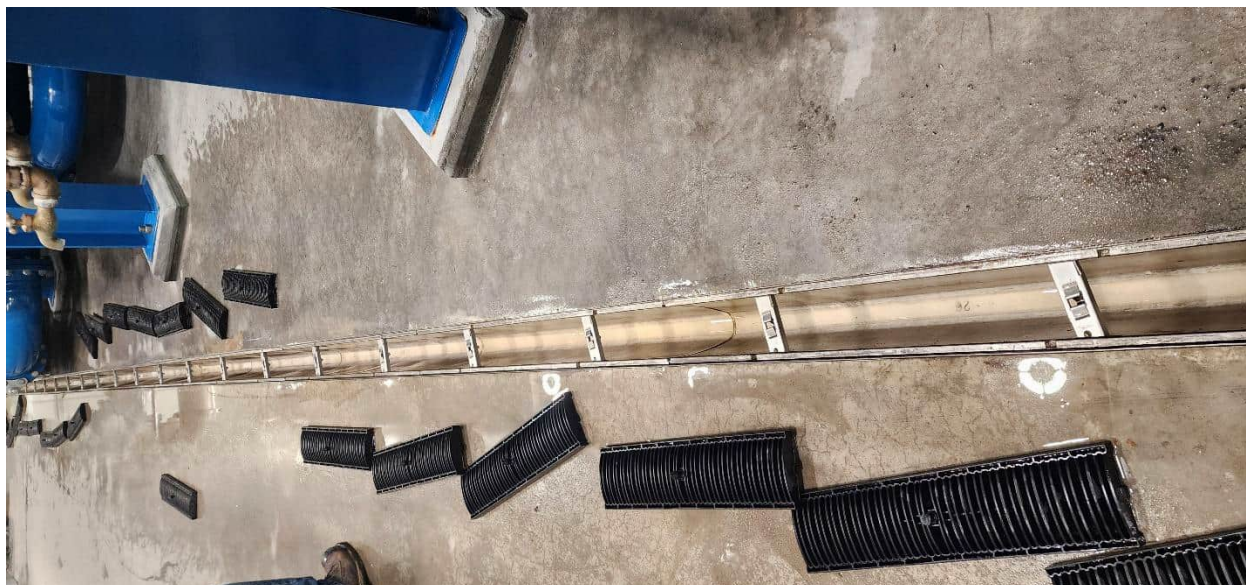
Checking southside trench drain in Structure 120 for any damage from acid spill used during Caustic Rinse of PFAS Vessel 5A
