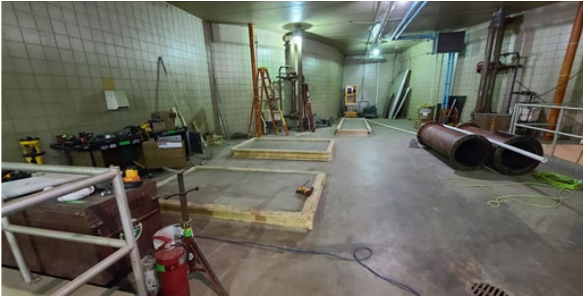
Structure 700 (Digester Building) boilers 1 and 2 equipment pads and the digester heat exchanger pad.
