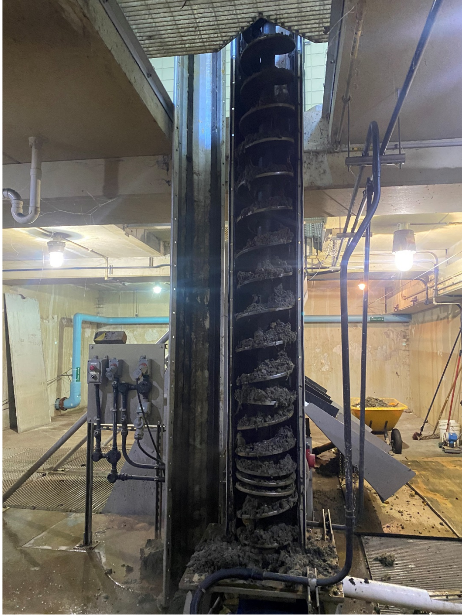
Sludge conveyor with side cover removed showing collapsed auger
