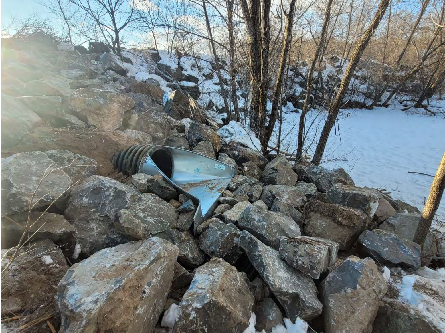
Stormwater detention area outfall piping
