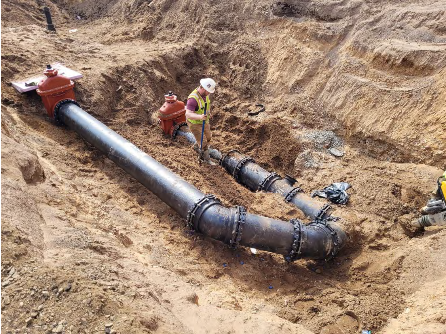
Well 10 bypass piping
