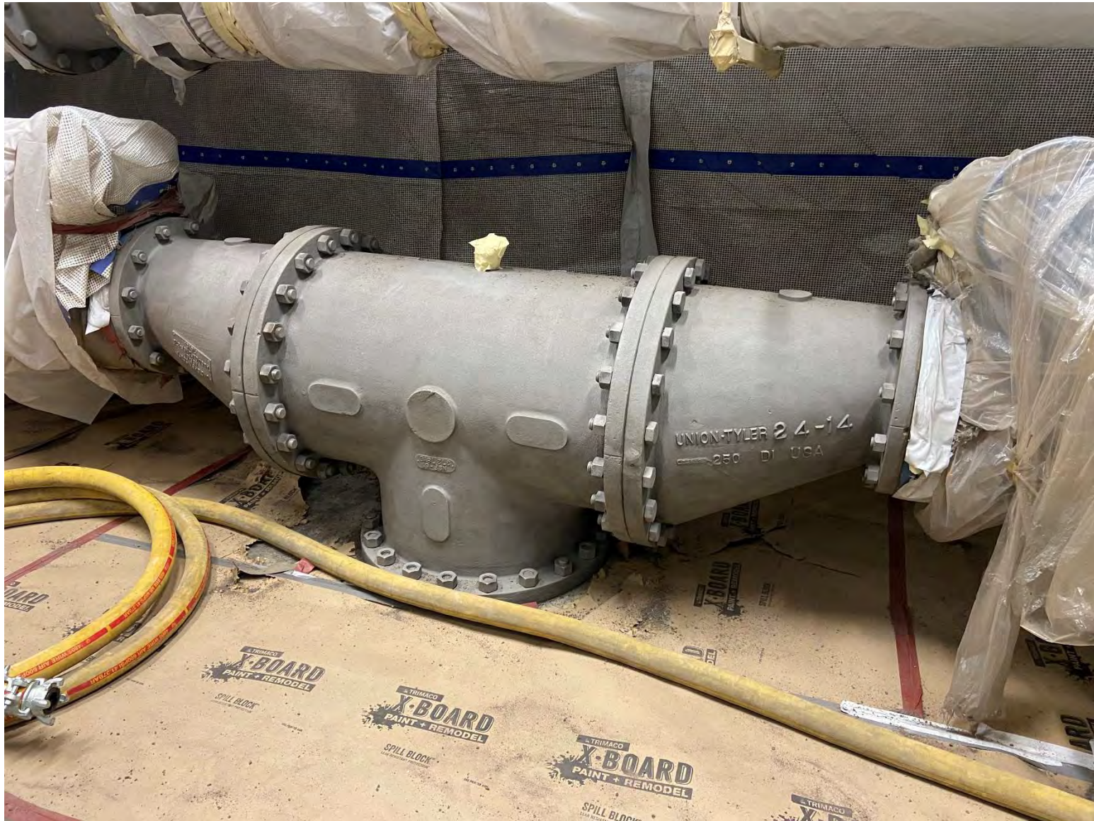
Treatment Facility – ductile iron pipe fittings with coating removed
