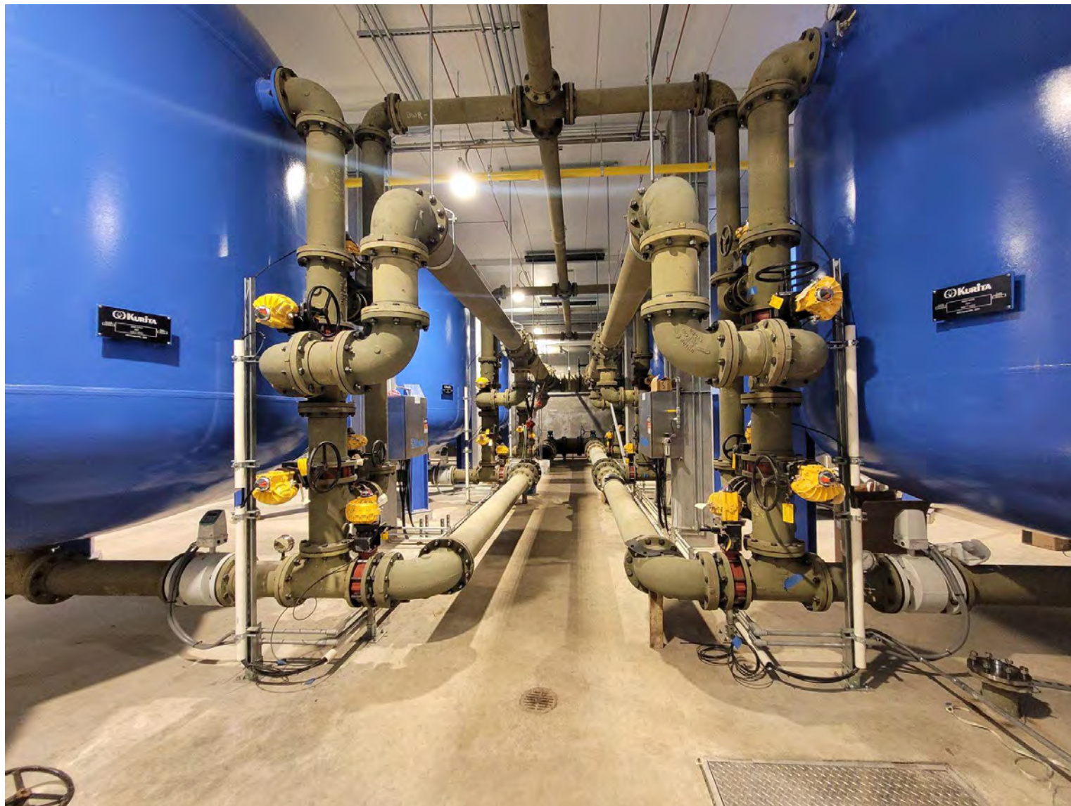
Treatment Facility – Anion Exchange tanks
