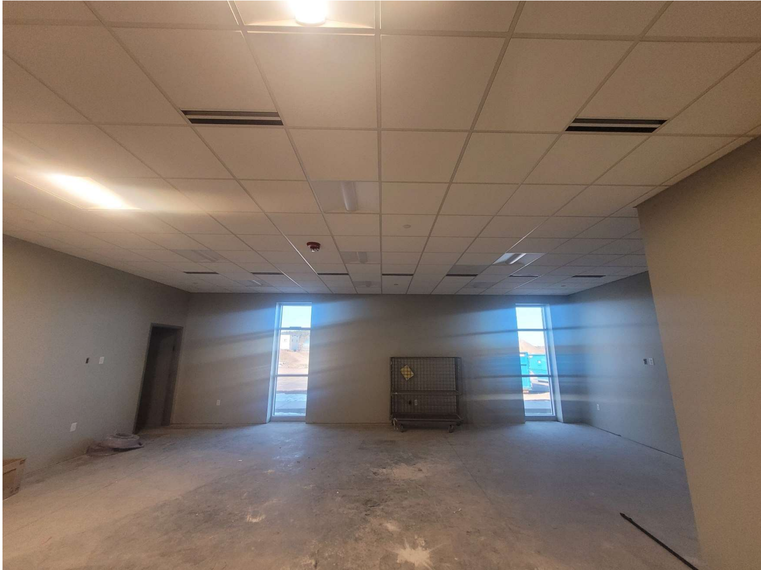
Admin. Bldg. – Ceiling tile
