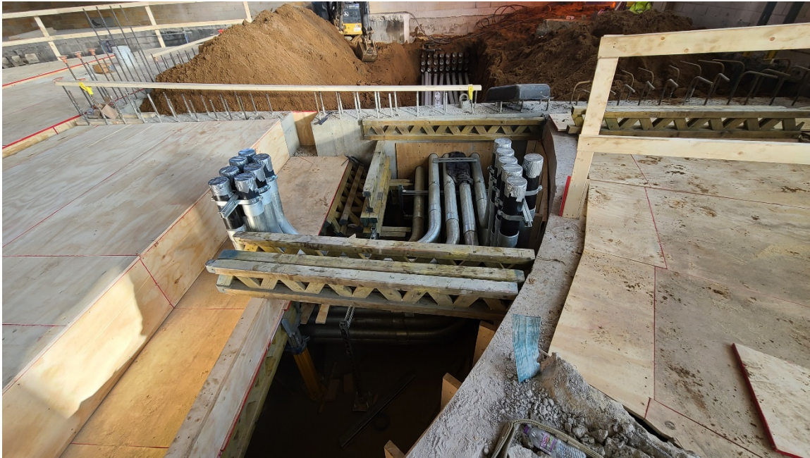
Conduit runs for new Structure 100 (Main Building) electrical switchgear
