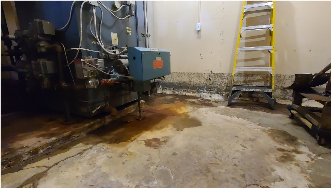
Line on wall in the Boiler Room of Structure 100 (Main Building), indicating sludge depth approximately 20 inches.
