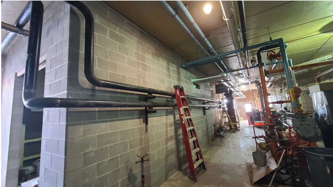
HWS and HWR lines installed and anchored to concrete masonry unit walls of electrical room in Structure 700 (Digester Building).
