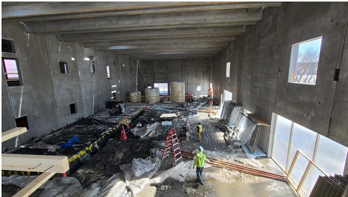
Looking east from the Control Room deck to the newly placed chemical feed tanks in Structure 770 (Solids Building).
