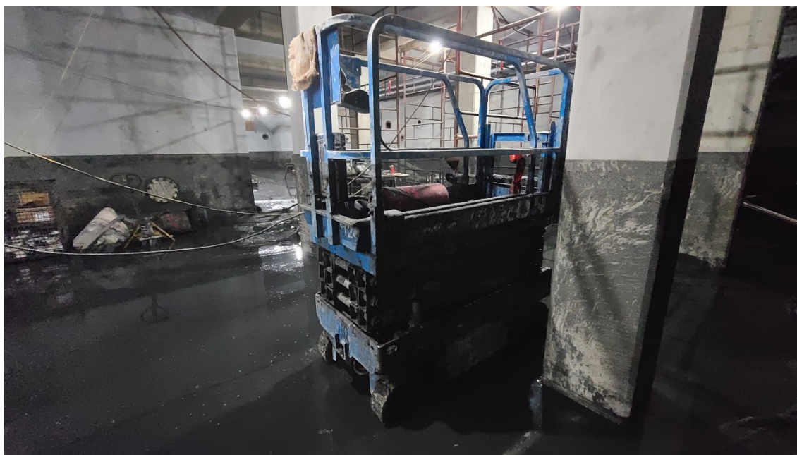
Sludge line on wall in the lower level of new Structure 770 (Solids Building) indicating sludge depth of approximately 56 inches.
