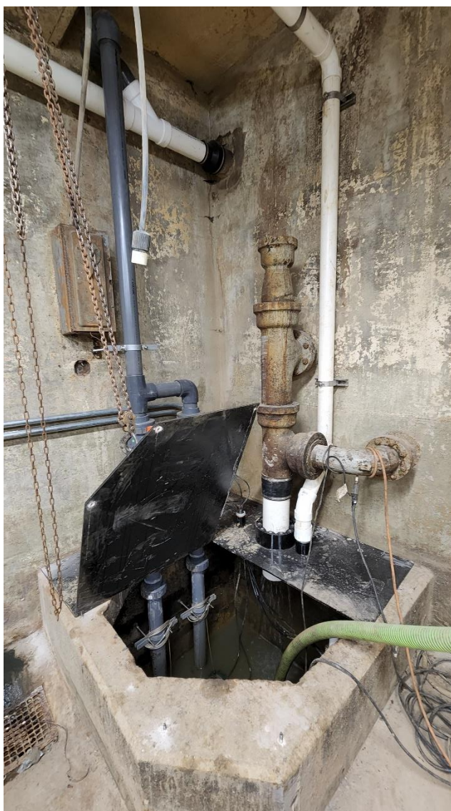
New lower level sump pumps, piping and cover at Structure 100 (Main Building).
