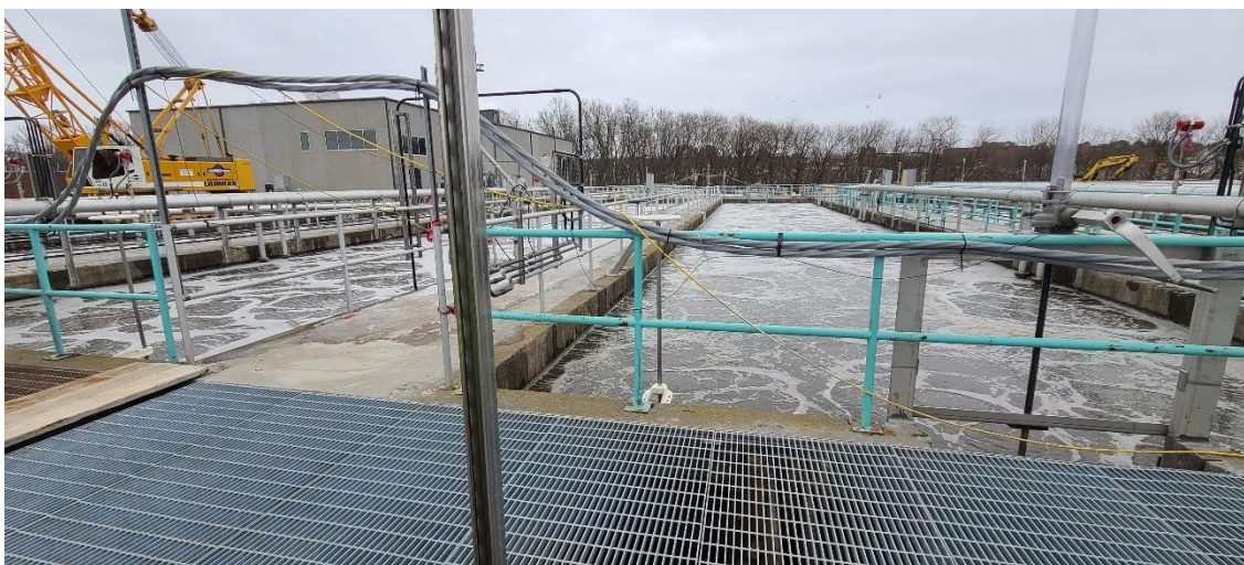
Structure 410 (Activated Sludge Basins): North Aeration Basins 1A, 1B and 1C in operation for first time with new equipment and diffusers.
