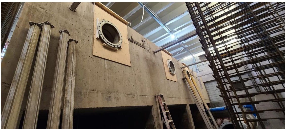
Inlet connection piping wall fittings to Disk Filters Structure 600 (Effluent Building).
