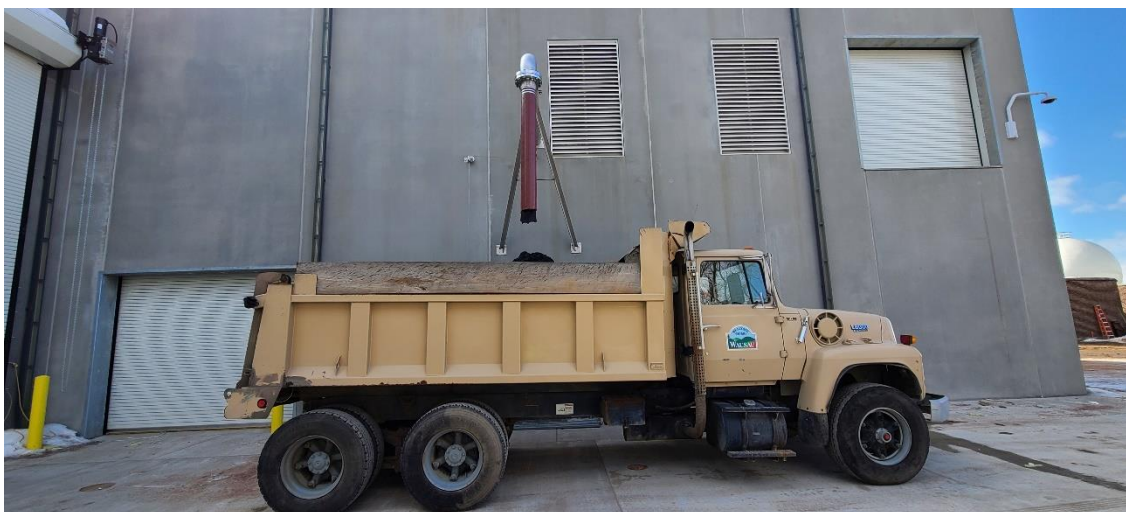
Receiving sludge from BFPs through sludge bypass line at Structure 770 (Solids Building).
