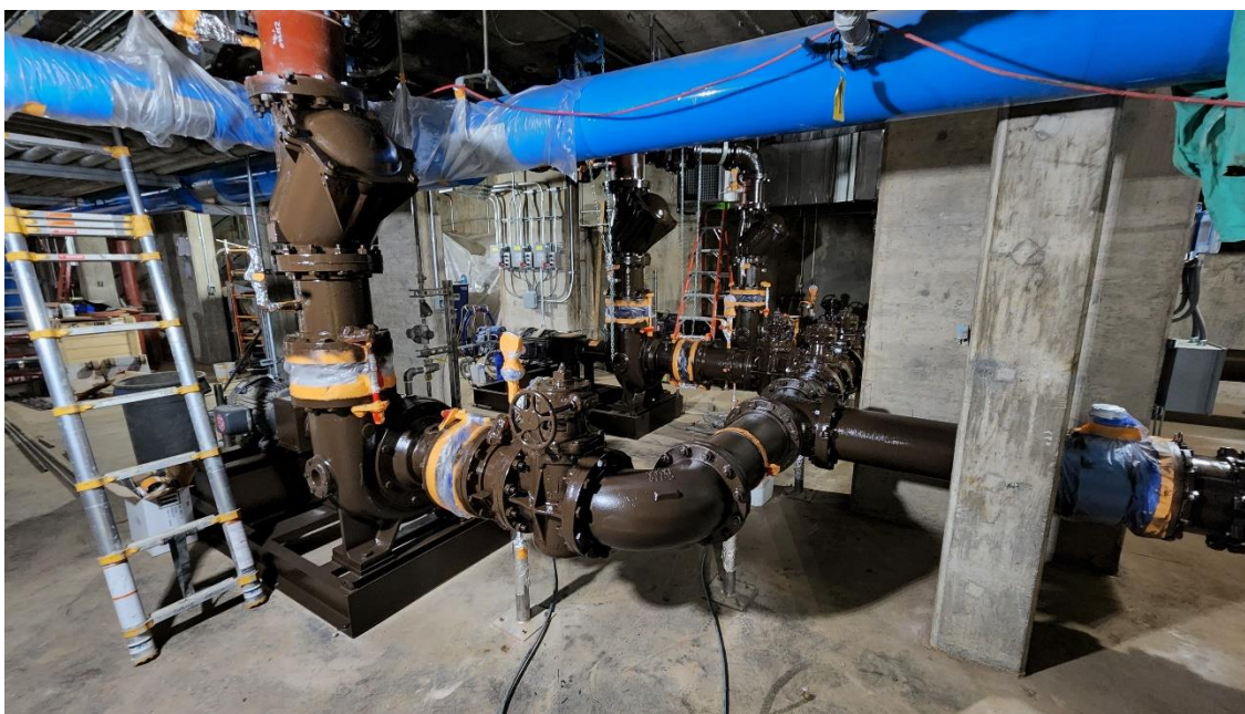
Structure 400 (Activated Sludge Building) painted return activated sludge (RAS) pumps and piping.
