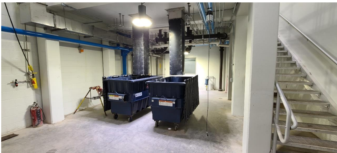
Sludge screen chutes and collection bins ready to receive primary screenings at Structure 770 (Solids Building).
