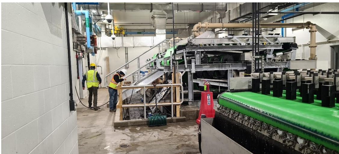
Charter Machine checking out and starting the belt filter presses at Structure 770 (Solids Building).
