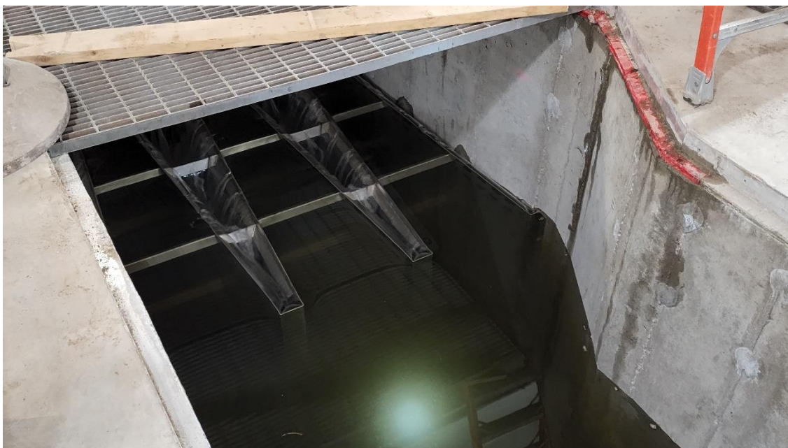
Plant effluent flow going over the UV channel weir for the first time at Structure 600 (Effluent Building).
