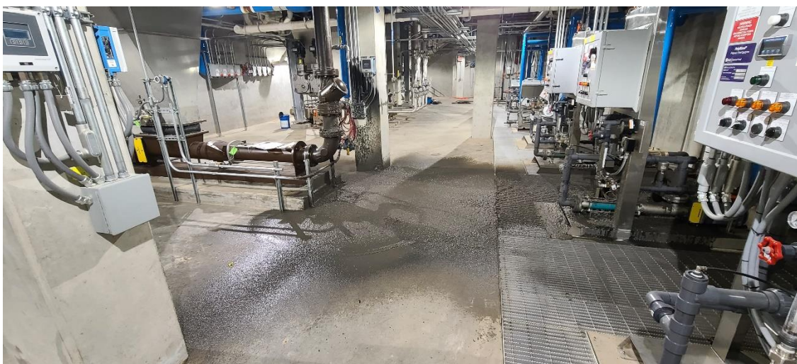
Structure 770 (Solids Building): unfortunately, sometimes leaks and messes occur during startup of new equipment.
