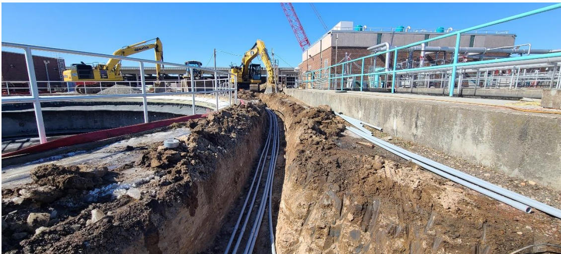
Conduit run for controls and power to Structures 510 and 520 (Secondary Clarifiers 1 and 2).
