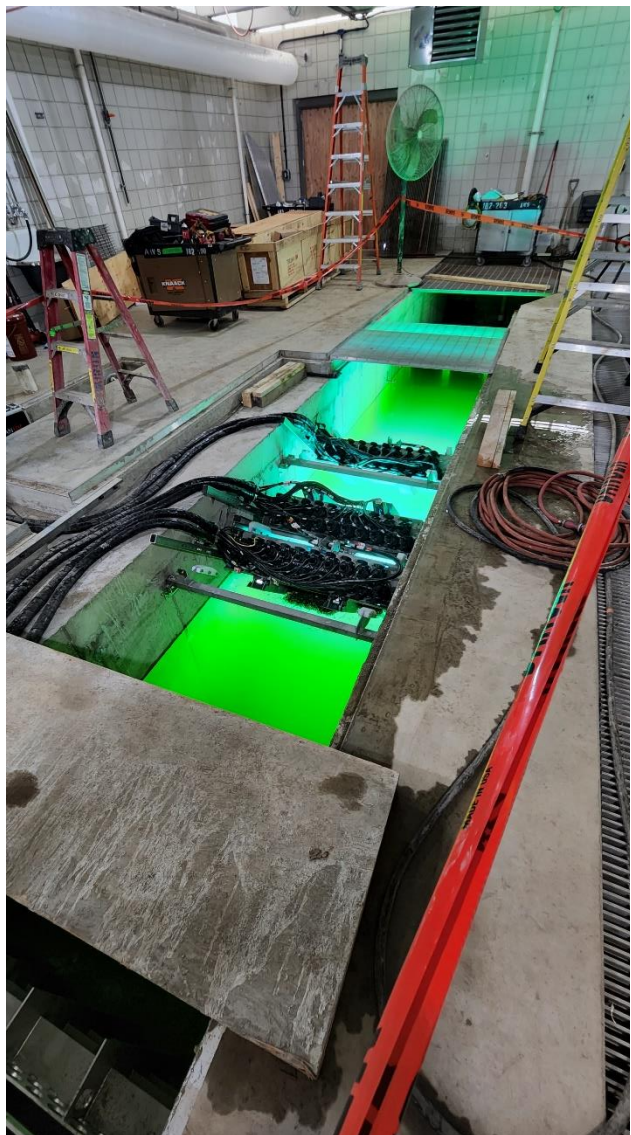
UV disinfection in operation at Structure 600 (Effluent Building).
