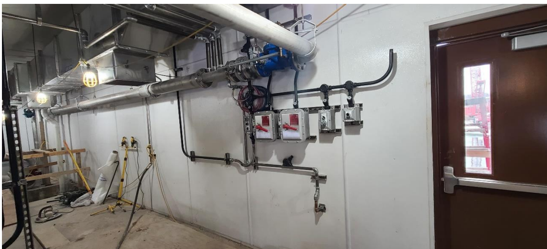
Grit pump and propeller equipment disconnects and HVAC duct work at Structure 200 (Grit Building).
