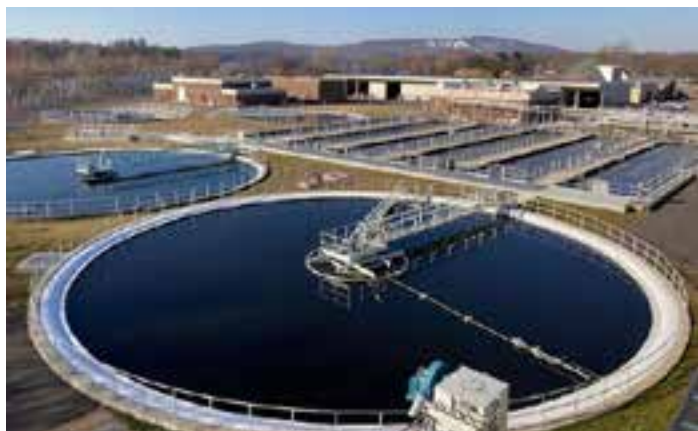
Secondaries and aeration basins
