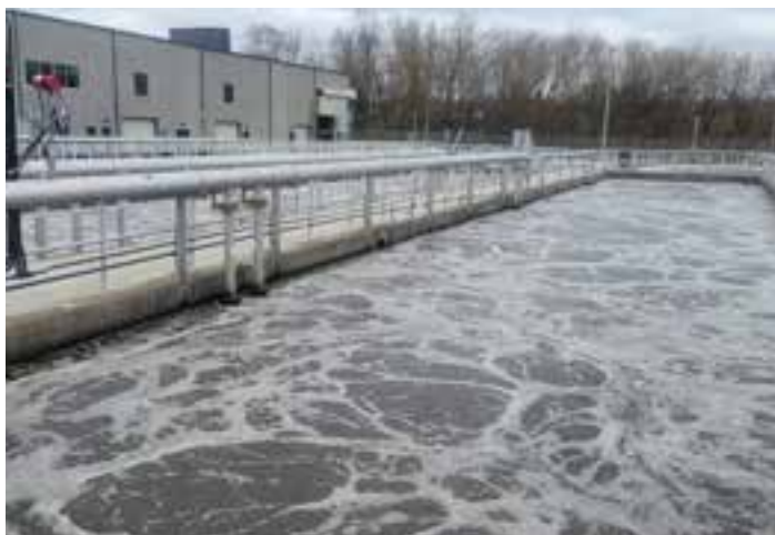
Dual drop leg aeration system
