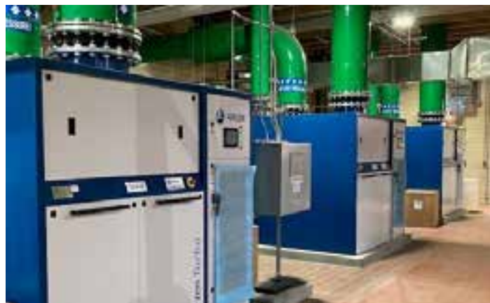
New Aerzen blowers
