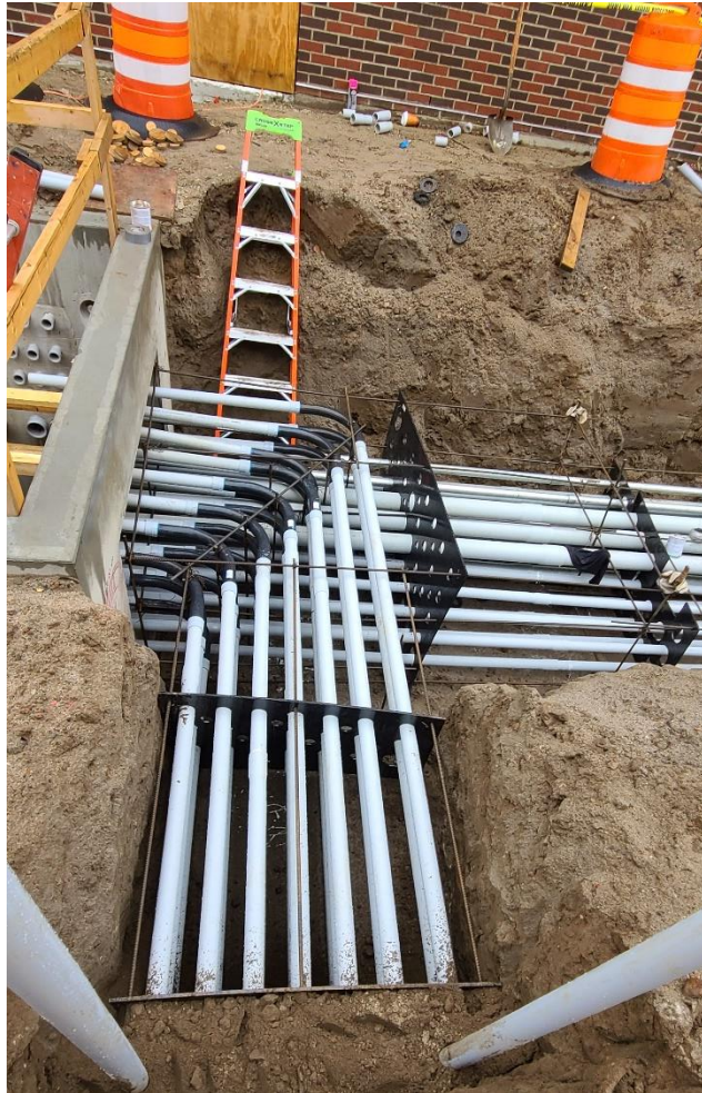
Portion of Duct Bank M and P coming out of the Electrical Manhole between Structure 600 (Effluent Building) and 610 (Chemical Building)
