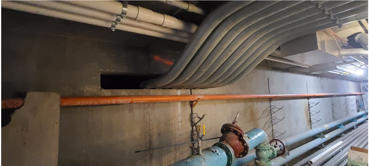
North end of Tunnel 900: 4-inch electrical conduit exiting the east tunnel wall to electrical manhole 1.
