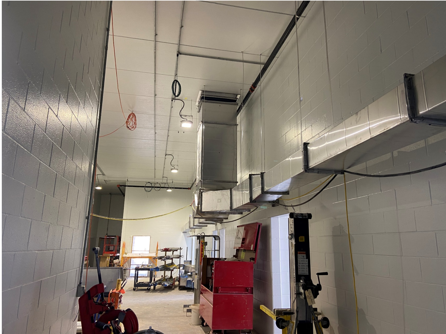
Maintenance Area 1 in the Process Building with HVAC, Electrical, Fire Suppression, and Coatings Installed
