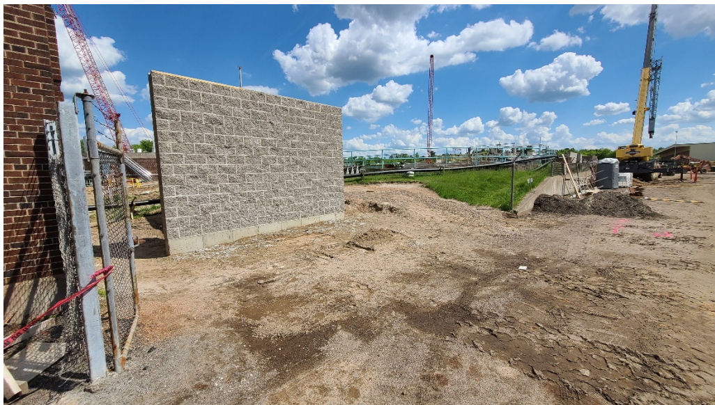
South transformer blastwall hiding Structure 105 (Standby Fuel Tank).
