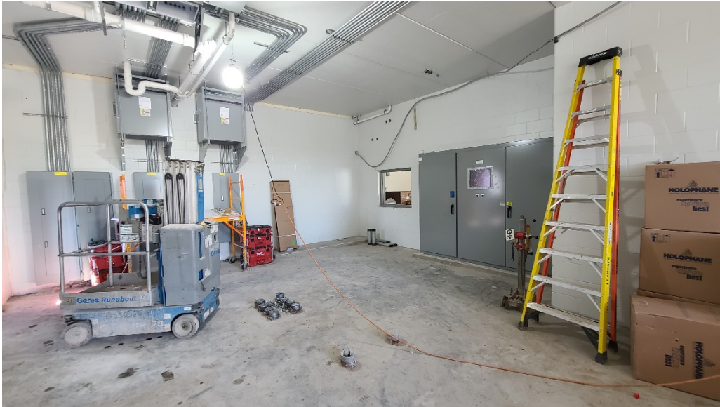
Electrical Room Structure 770 (Solids Building, showing the newly set Dryer LCP to the left of the ladder).
