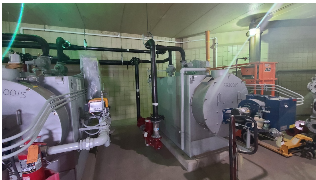
New boilers and piping.
