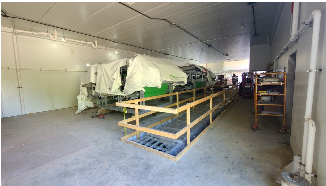
Belt presses, gravity belt thickeners and TWAS hopper set in Structure 770 (Solids Building).
