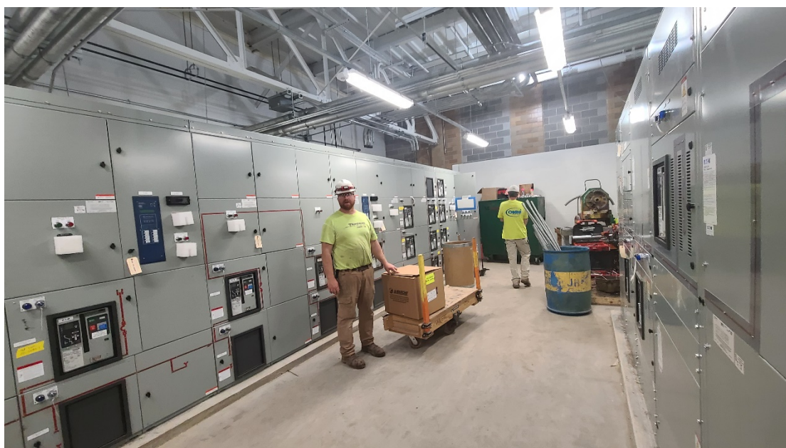
New switchgear and switchboard in electrical room.
