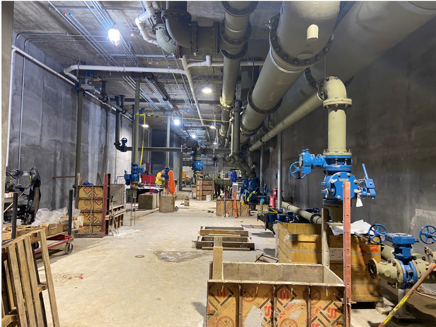
Lower Level Process Piping and Equipment
