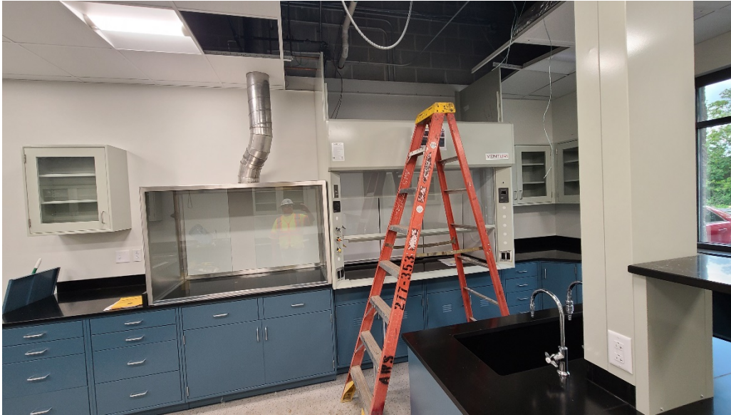
Exhaust hoods and new lab benches and cabinets.
