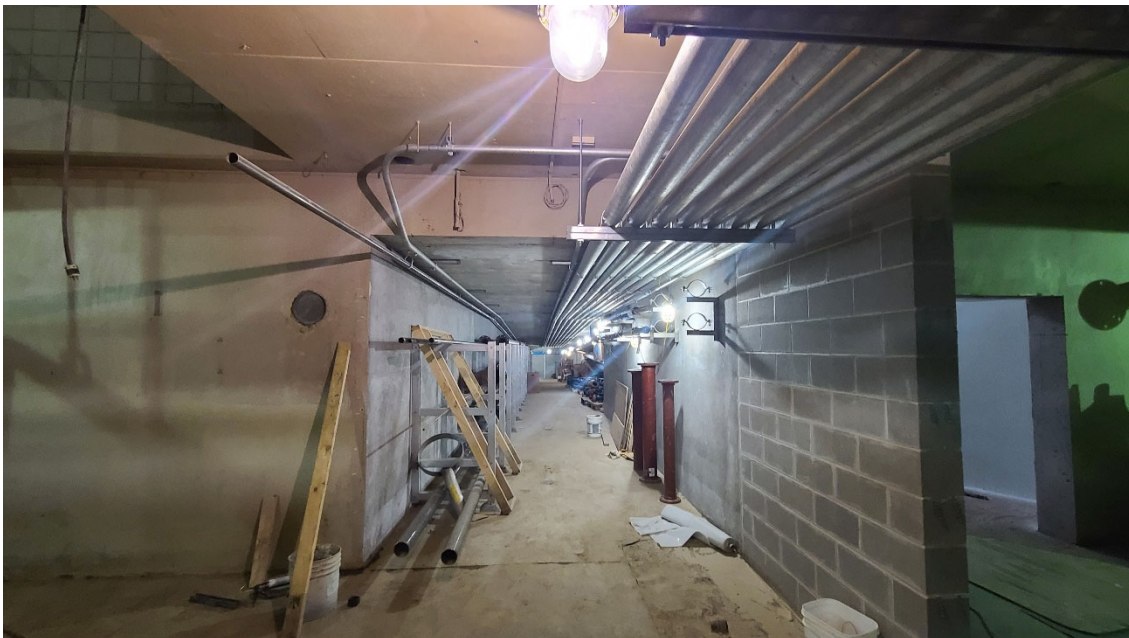
North end of tunnel looking south down Tunnel 910 with electrical conduit runs overhead.
