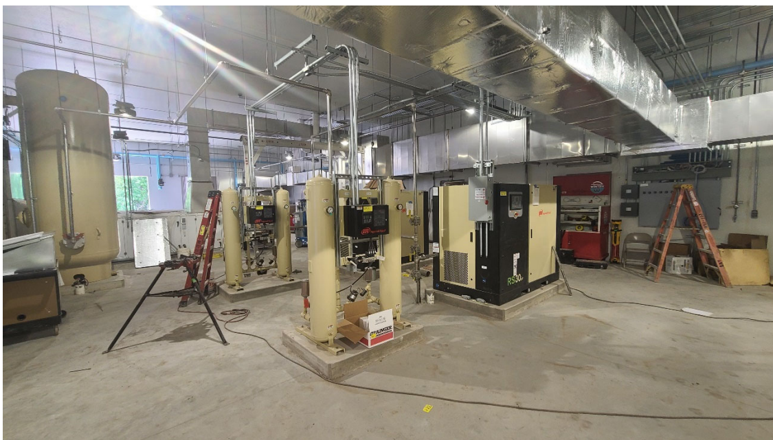
Structure 770 (Solids Building) upper mechanical room, showing desiccant dryers and air compressors with associated receiver tank
