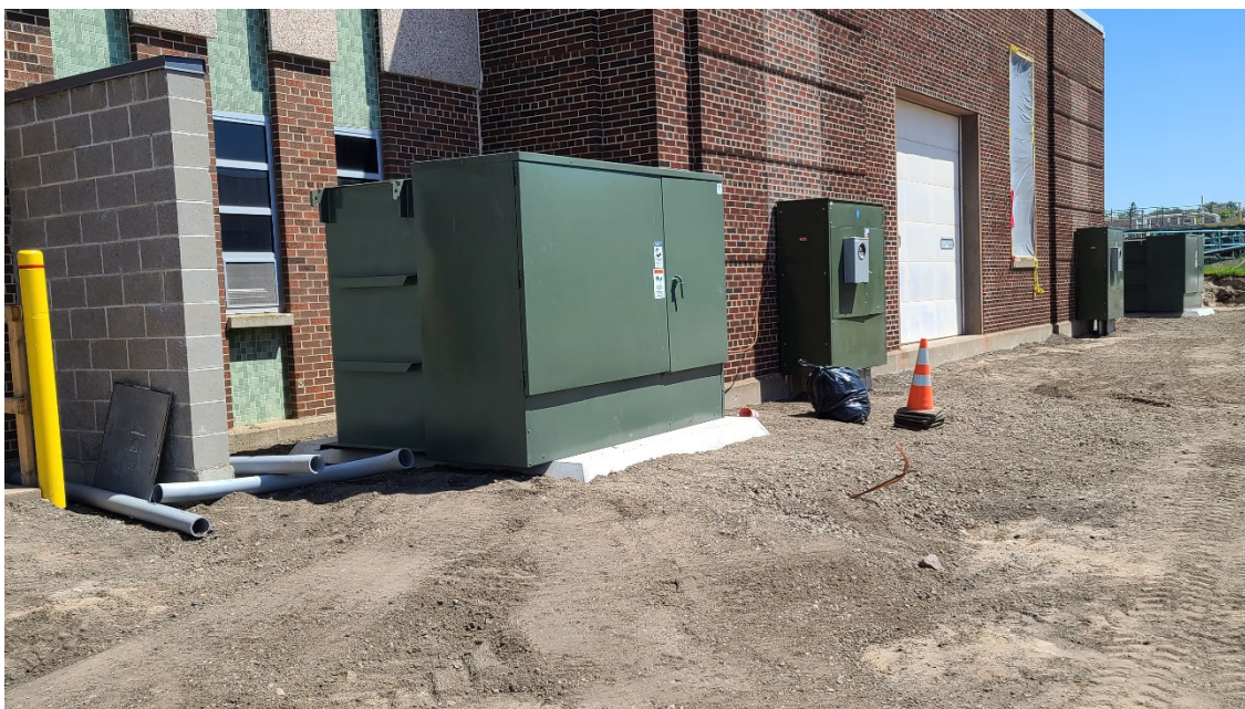
New main feed transformers set on west side of Structure 100 (Main Building).
