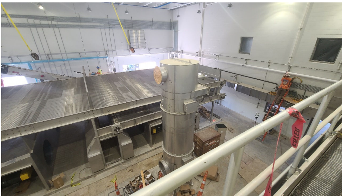
Looking down from catwalk of Structure 770 (Solids Building) at the west side of the new dryer and condenser tank.
