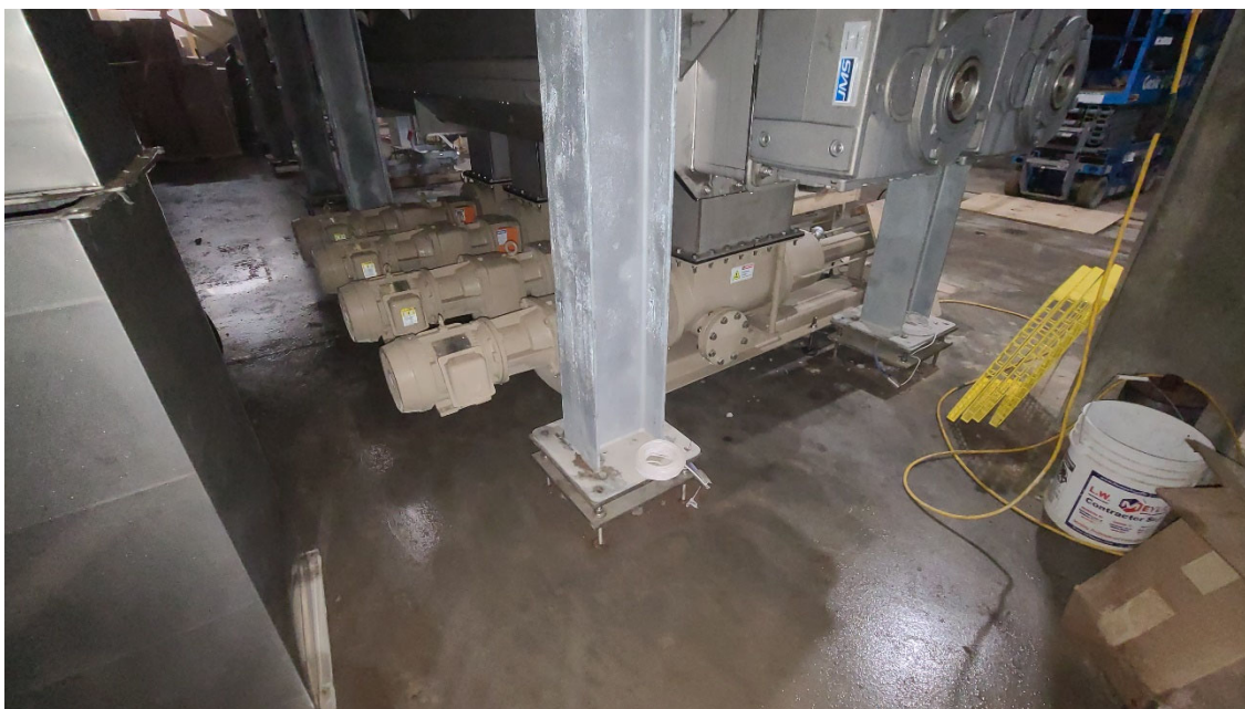
New cake hopper progressive cavity pumps in the lower level of Structure 770 (Solids Building).
