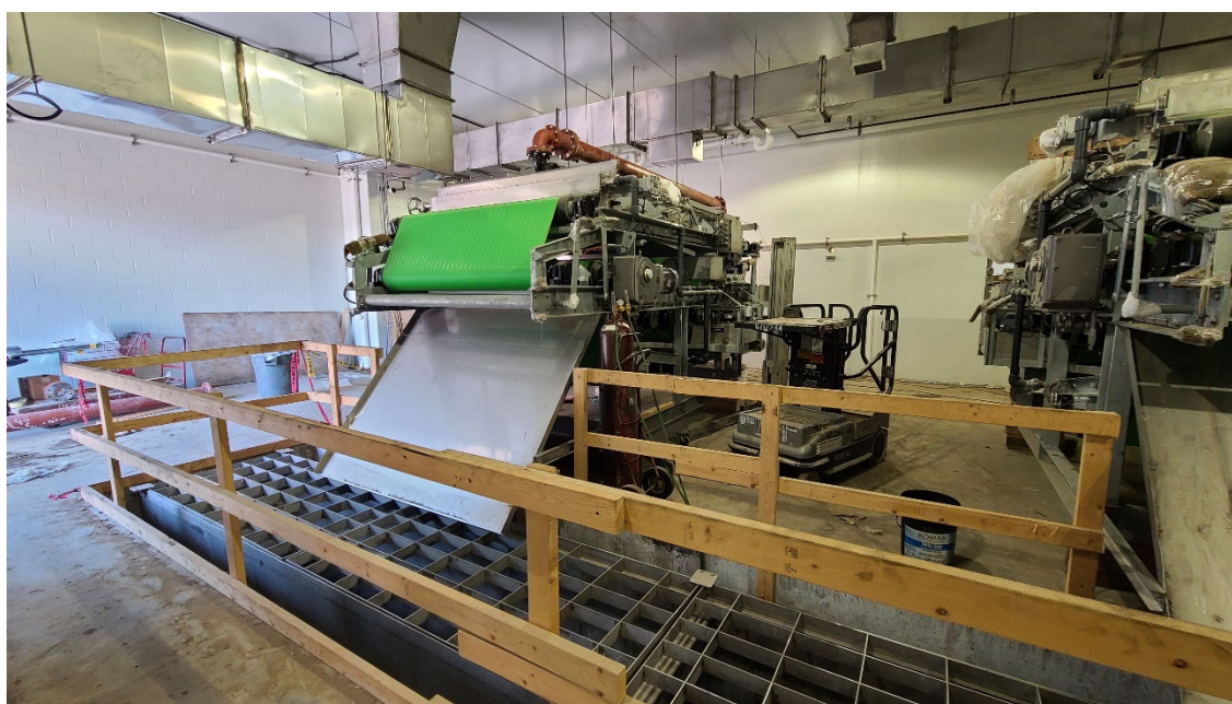
Structure 770 (Solids Building) belt filter press set with chute to cake hopper.
