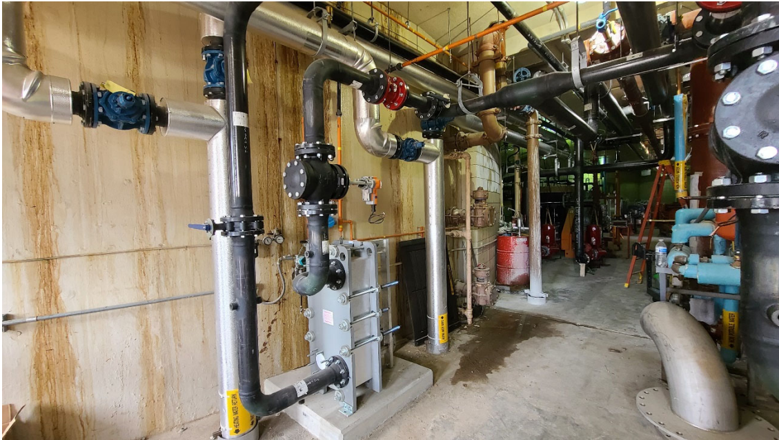
Heating water supply and return piping to Structure 710 (Digester 1) heat exchanger.
