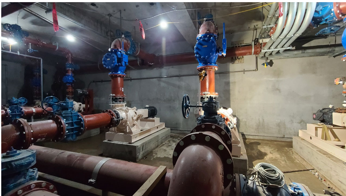
New return activated sludge pumps and associated piping in lower level of Structure 770 (Solids Building).
