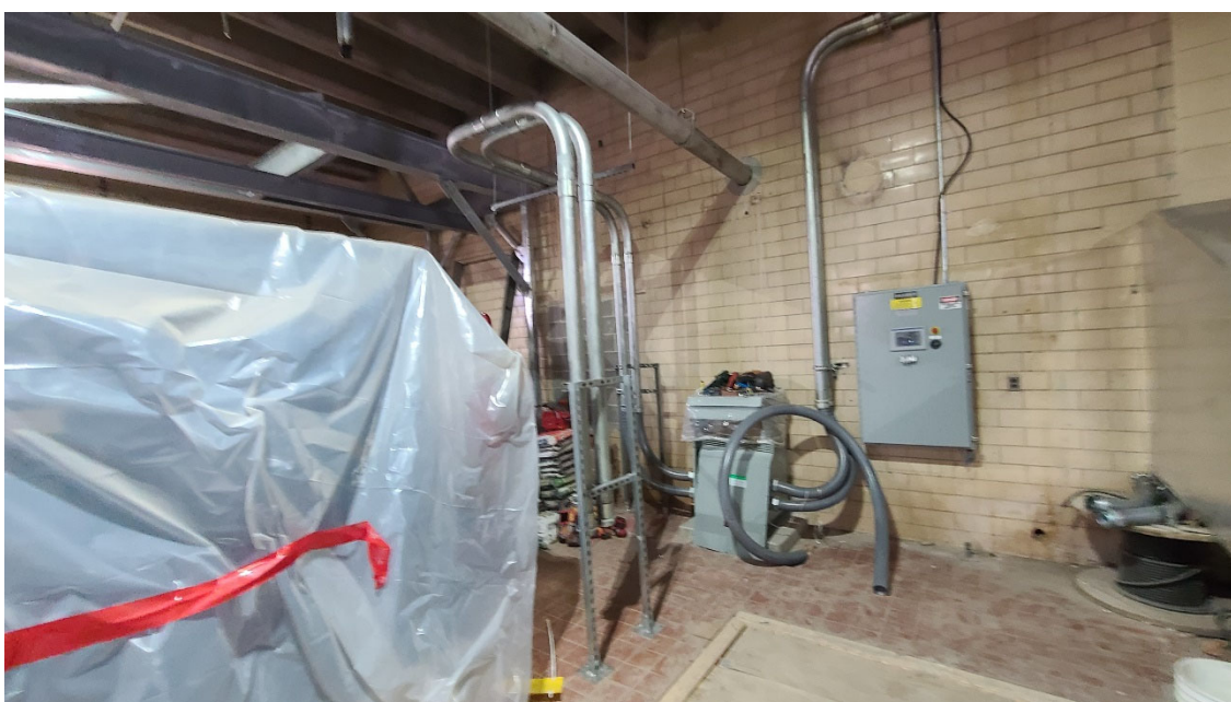
Conduit for new north blower and harmonic filter at Structure 400 (Activated Sludge Building).
