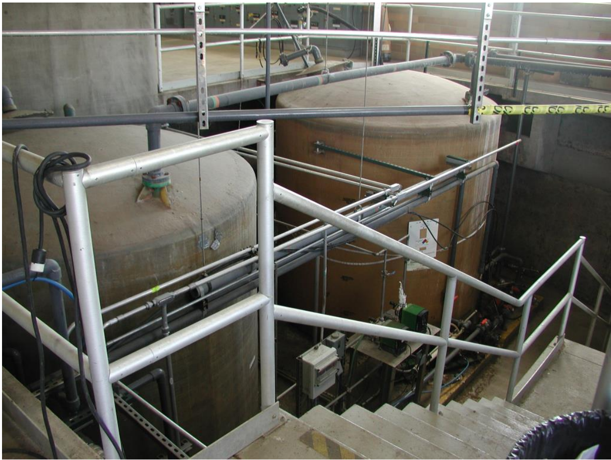
Photo 7: Alum tank on left, Polymer tank on right
