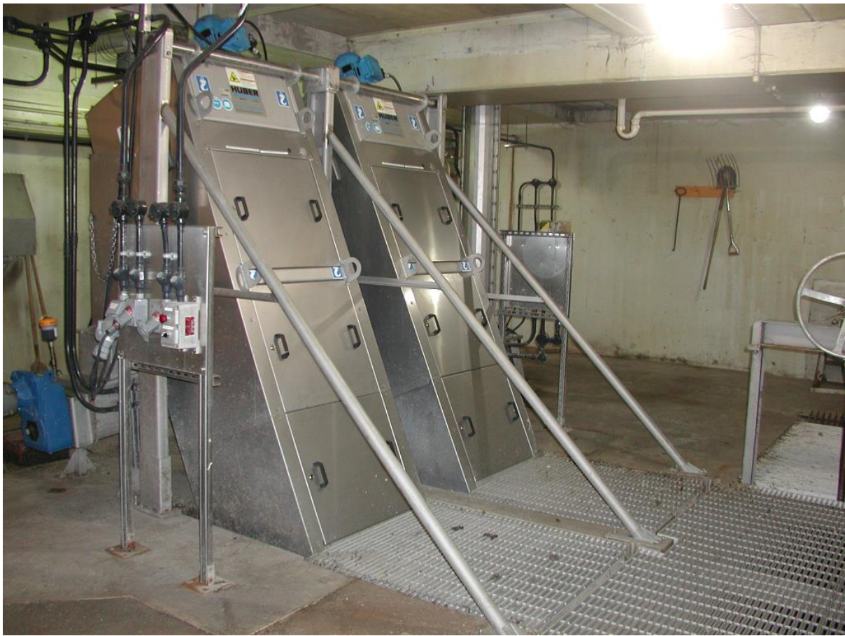
Photo 3: Dual influent travelling bar screens
