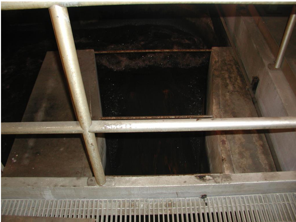
Photo 10: Influent Parshall flume (downstream)
