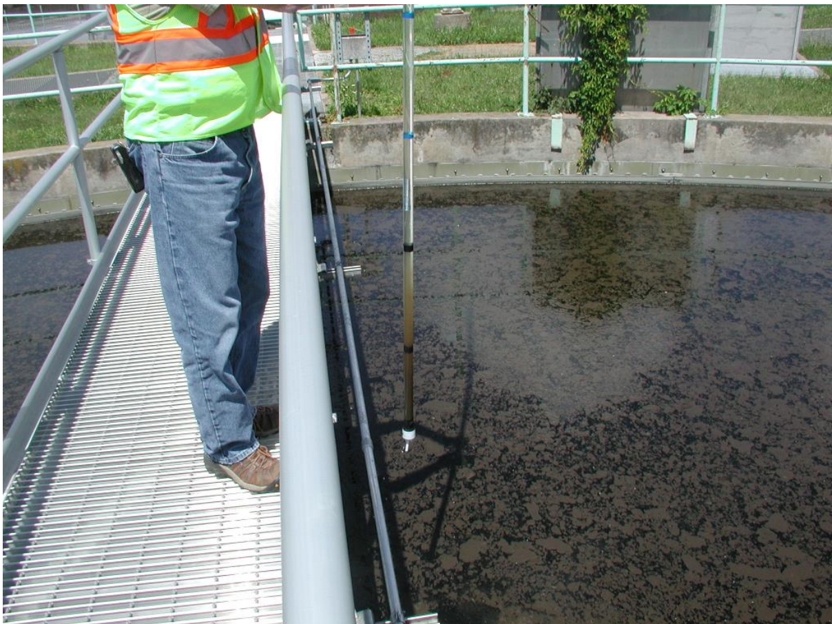
Photo 18: Southeastern secondary clarifier sludge depth
