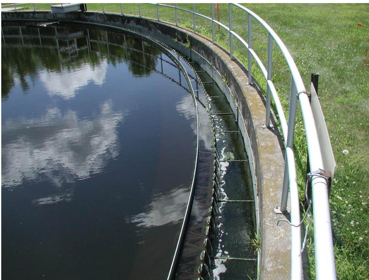
Photo 14: Secondary clarifier effluent weir and trough.
