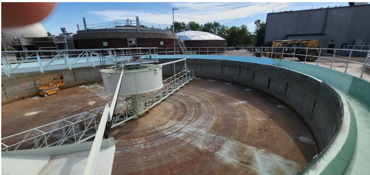
Mechanism installed, launder trough coated for Structure 320.
