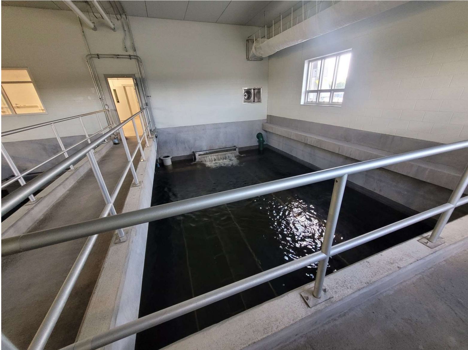
Water Filter in Operation
