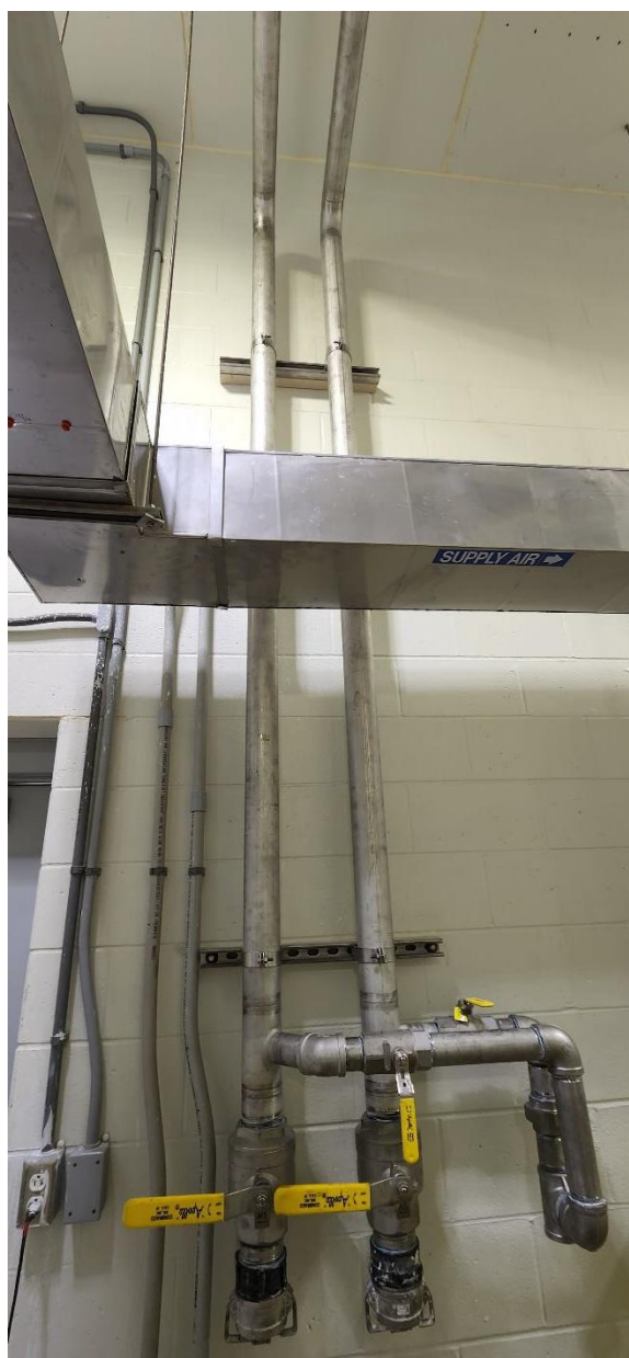
New Magnesium Hydroxide Solution (MHS) stainless fill connection piping and valves at Structure 610 (Chemical Building).
