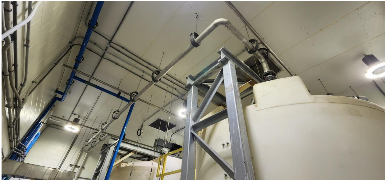
Stainless fill piping tank connections for MHS at Structure 610 (Chemical Building).
