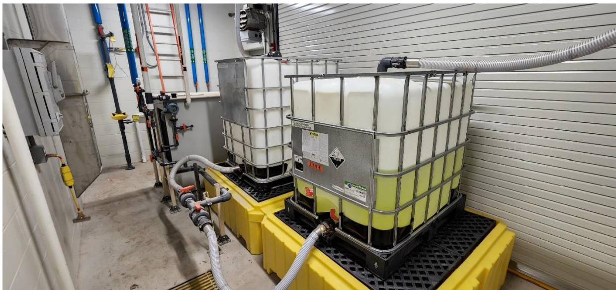
The correct tote storage containment racks arrived for the sodium hypochlorite (SHC) System at Structure 610 (Chemical Building).
