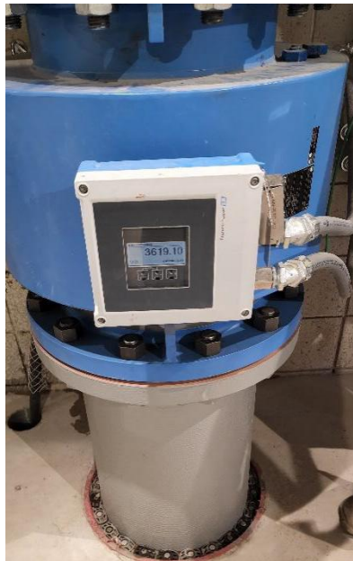
Secondary effluent pump in operation, new flow meter readout at Structure 600 (Effluent Building).
