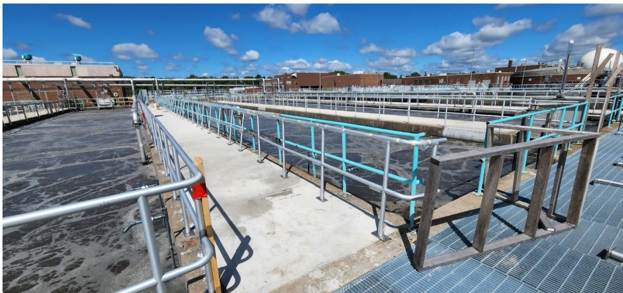
Activated sludge basins in operation and working well.
