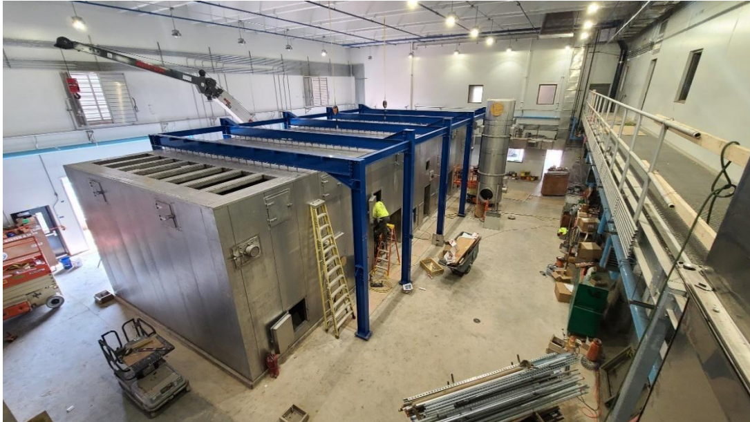
Looking down from catwalk at the north side of the new dryer and condenser tank of Structure 770 (Solids Building).
