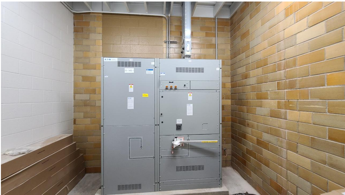
Inside Electrical Room 2 with new Switchboard and bus duct of Structure 100 (Main Building).
