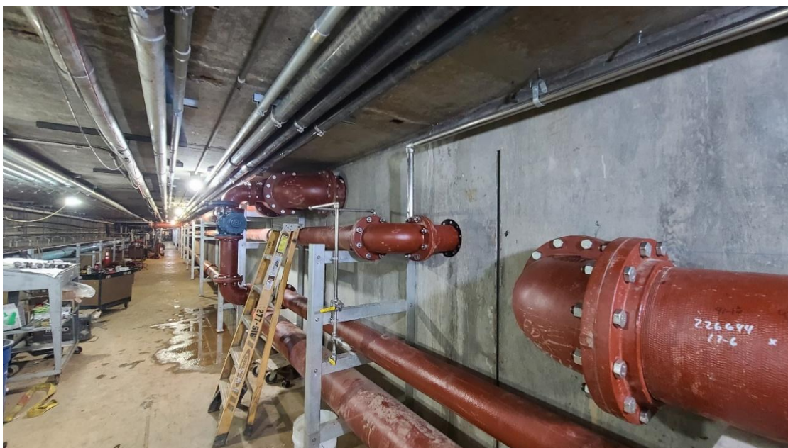
Looking east about mid Tunnel 900 at the RCY, SSM and RAS lines that exit/enter the tunnel from the east.
