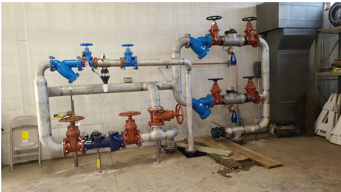
New backflow prevention for plant in Structure 110 (Vehicle Storage Building).
