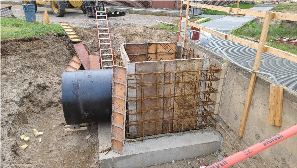
Pipe sleeve for small manhole/vault structure between Structures 510 and 520 (Secondary Clarifiers).
