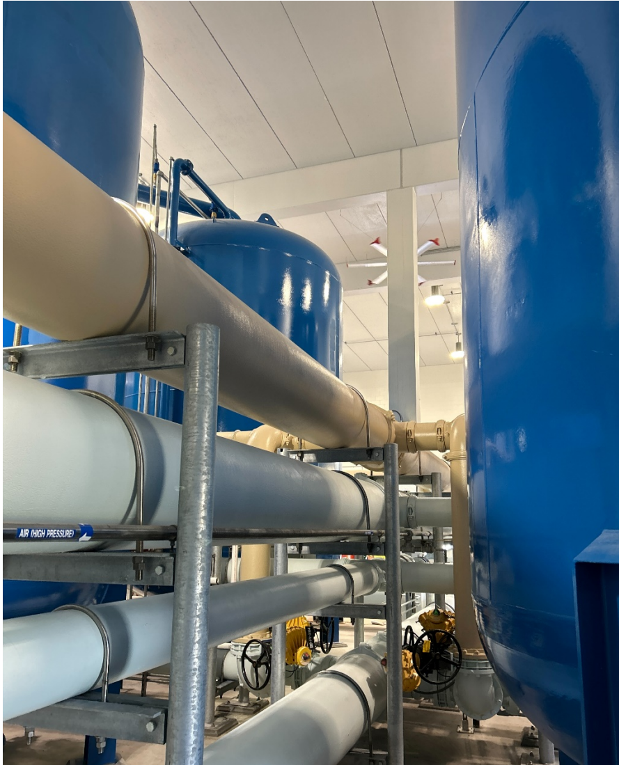
PFAS backwash influent and effluent and PFAS influent and effluent piping along with actuated valves in Structure 120.
