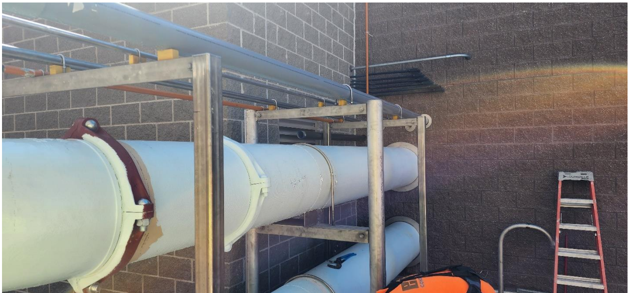
20-in PFI and PFE lines through wall of Structure 100 (Process Building).
