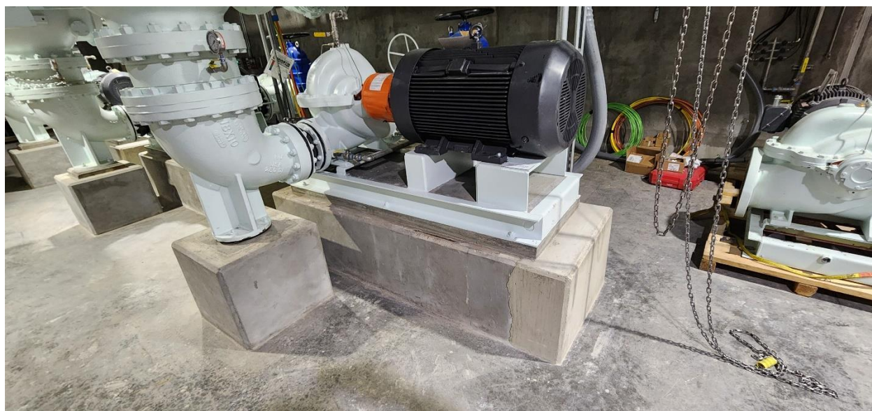
Filtered Water Pump 3 installed, tested and operational.
