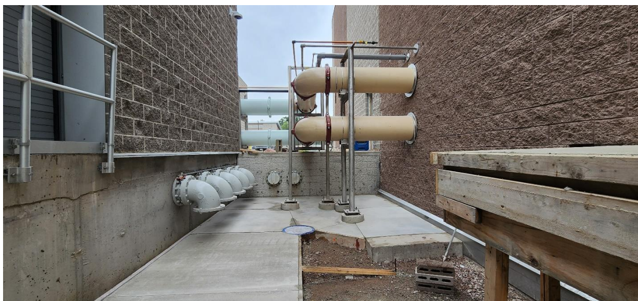
Piping stack between Structure 100 (Process Building) and entering Structure 120 (PFAS Treatment Building) on right, looking west with overflow piping from Structure 100 shown on left.
