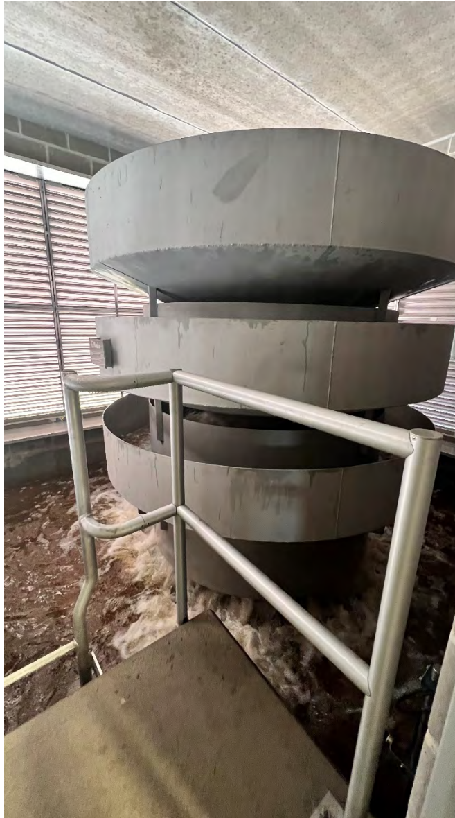
Gravity Aerator under Maximum Design Flow
