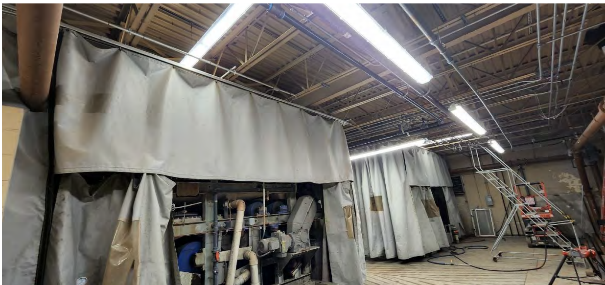
New lighting installed in old belt filter press room of Structure 100 (Main Building).
