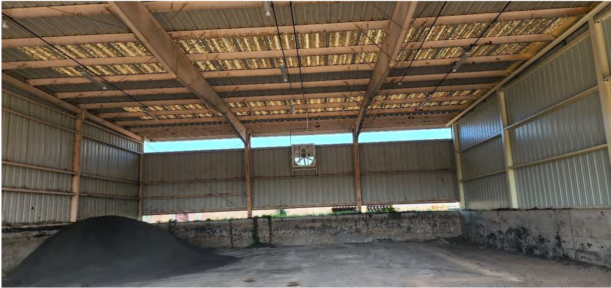
New south bay exhaust fan installed at Structure 760 (Biosolids Storage Building).
