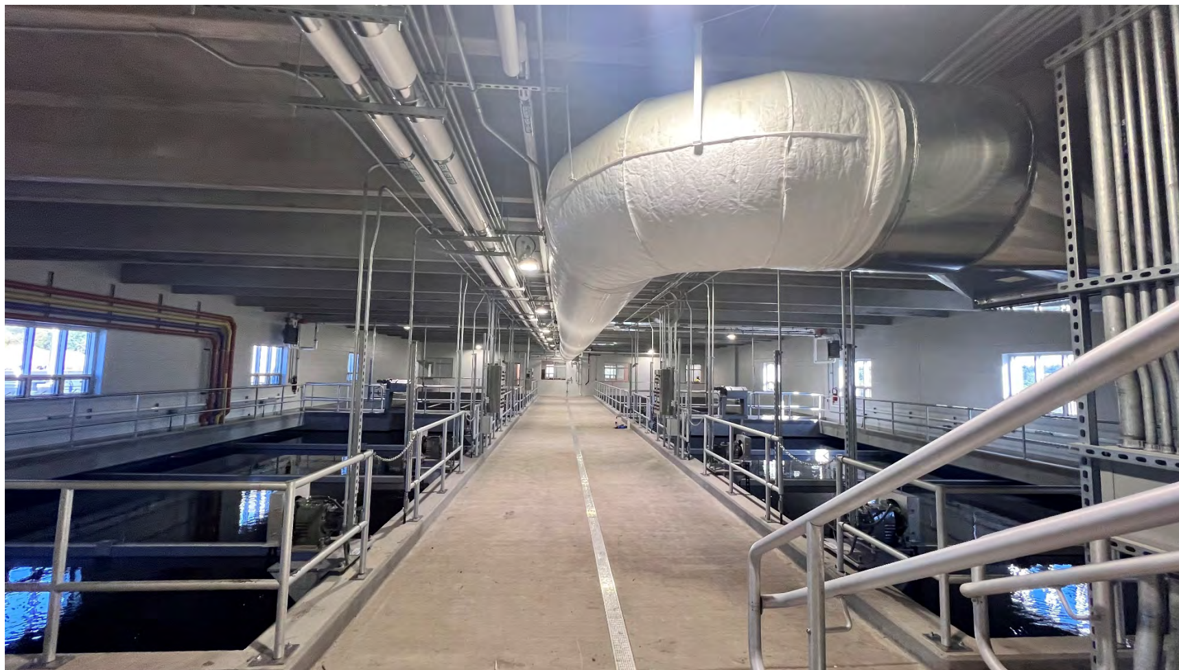
Chemical Addition and Settling Basins
