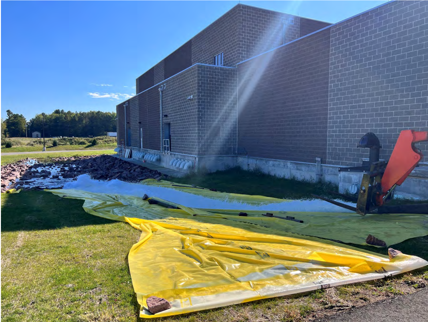
Temporary discharge of water to site storm water facilities
