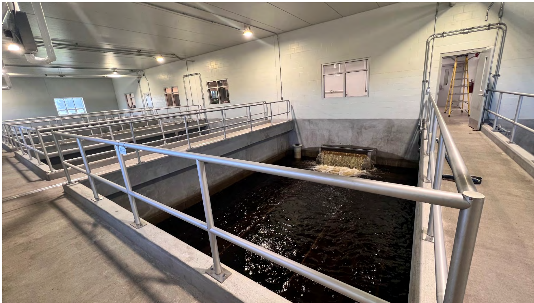
Filter Operation at Maximum Design Flow
