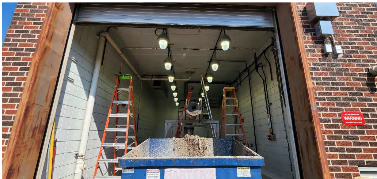
New lighting in screen/conveyor room of Structure 100.
