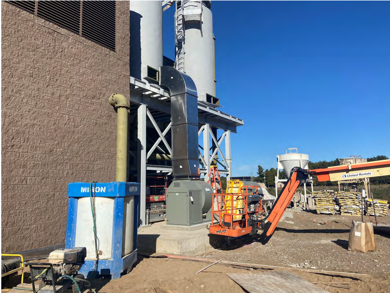
Air Strippers and Blower Units Located on Southeast Corner of DWTF
