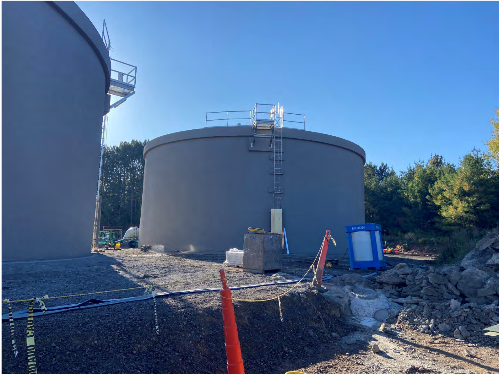
Clearwell Tanks, looking Southeast
