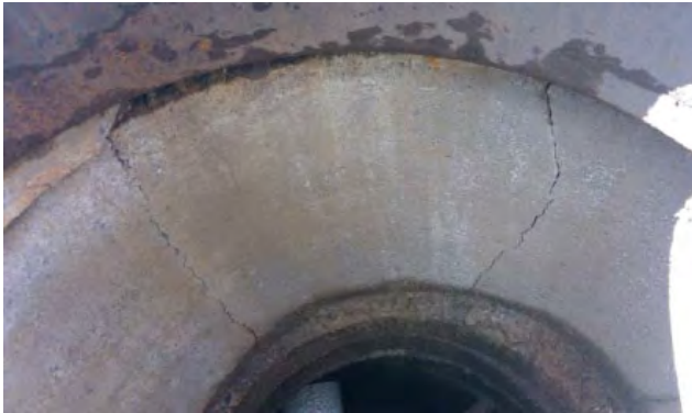
Cracking in Precast Chimney (smh1924)
