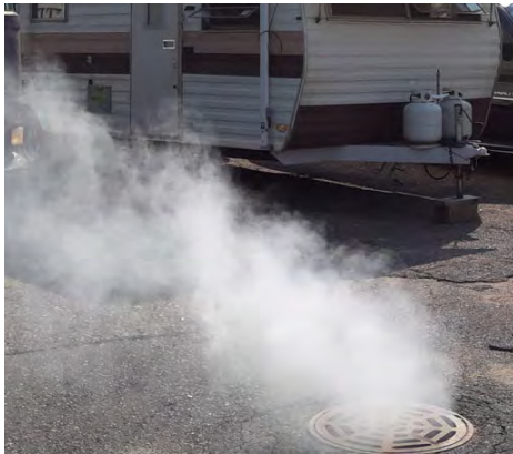
Smoke Exited Several Storm Covers in the Area
