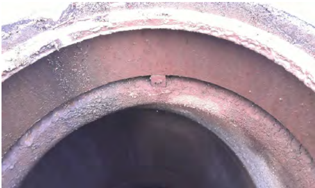
Shim Used for Manhole Adjustment (smh2393)
