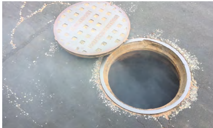
Smoke from Access Hatch Seals in Storm Sewer on 4th Ave. and 6th Ave.
