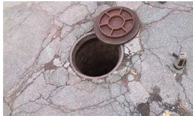
Pavement Cracking/Cover Gasket (smh2508)
