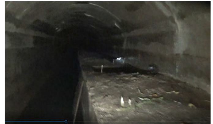
First Street Access Hatches Assessed in 2020 Noted Defects
