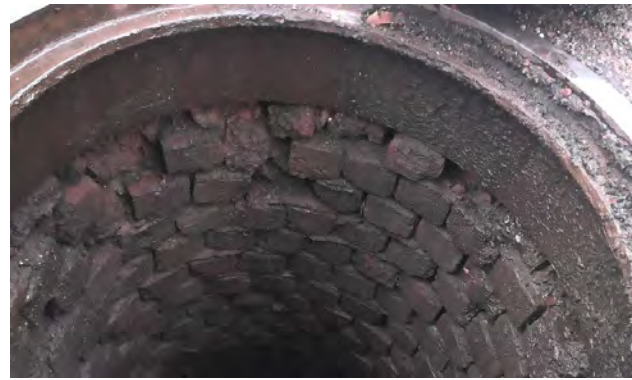
Broken Chimney (smh2424)
