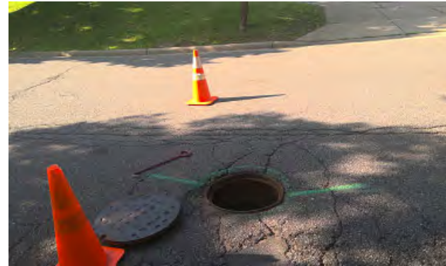
Surface Cracking and Depression (smh6603)
