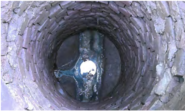
Missing Bricks and Mortar (smh3265)
