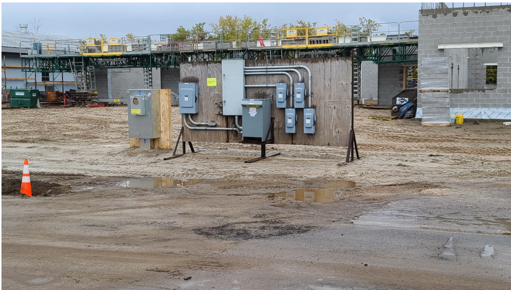
Temporary power setup for Structure 120 (Administration Building), waiting to get connected.
