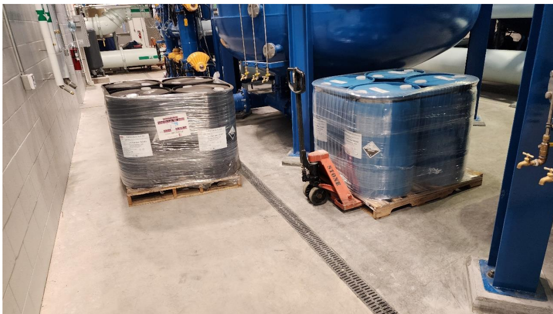
50% NaOH and 31.5% HCl onsite for Caustic Wash/Disinfection of PFAs Vessel 5A in Structure 120 (PFAS Treatment Building).
