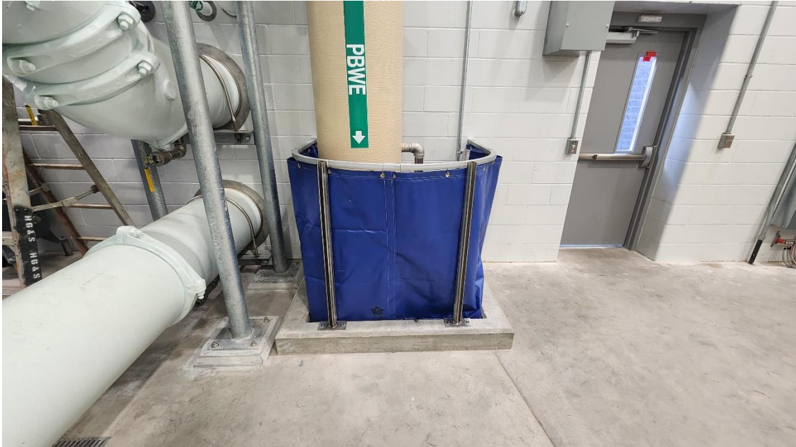
PFAS Backwash sump curtain installed in Structure 120 (PFAS Treatment Building).
