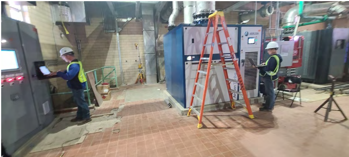
Donohue and Aerzen working in Structure 400 (Activated Sludge Building) for Blower #1 startup.
