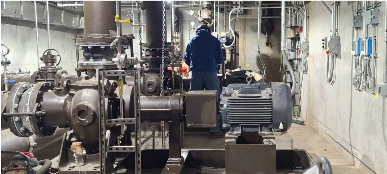
Structure 770 (Solids Building) return activated sludge pumps in lower level being checked out and started by the vendor.
