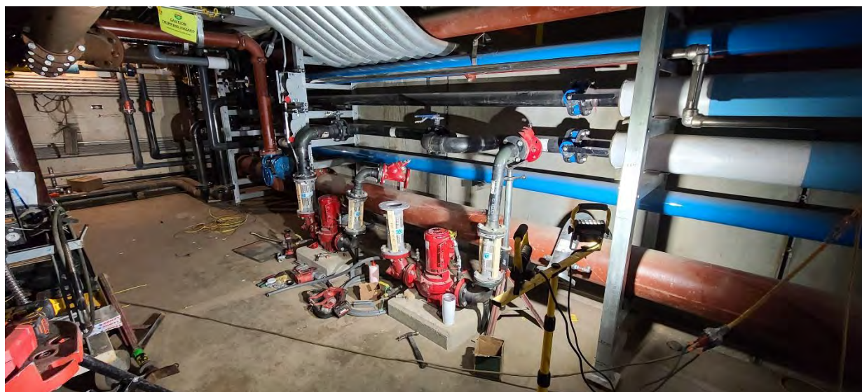
Hot Water Return/Supply Pumps set in Tunnel 900.
