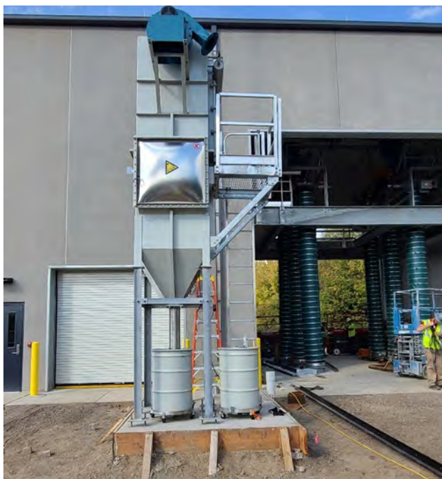
Structure 770 (Solids Building) dust collection system has been installed.
