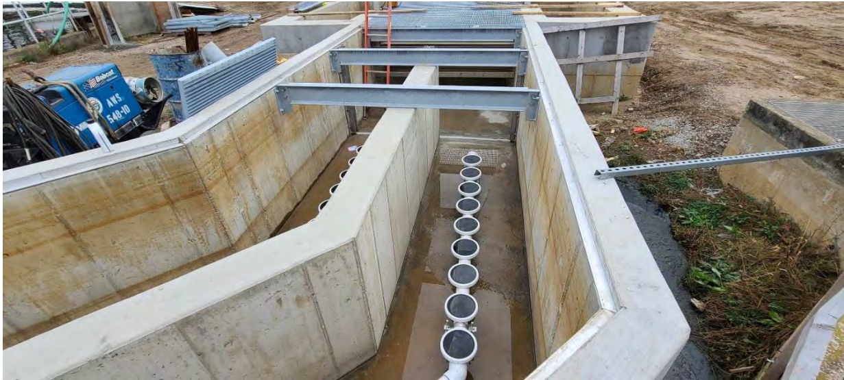
Aeration headers prior to entry into Structure 500 (Secondary Splitter).
