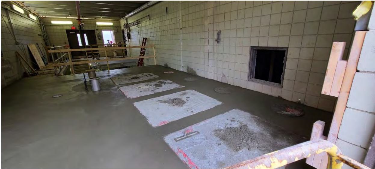
New Secondary Effluent area hatches for the pumps to be placed below at Structure 600 (Effluent Building).
