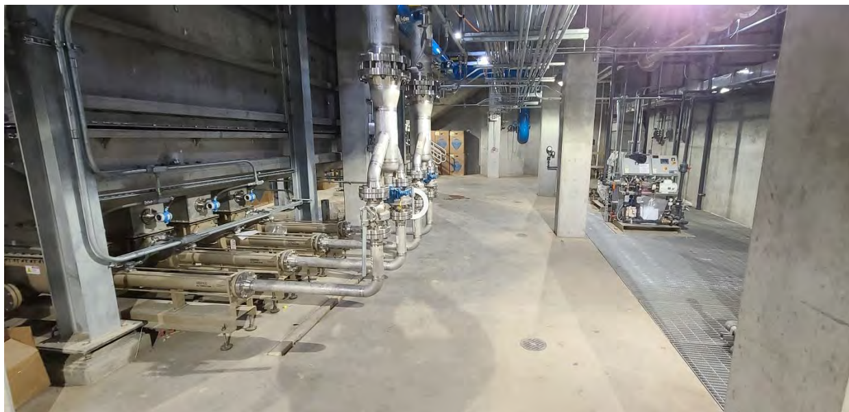
Lighting in the lower level of Structure 770 (Solids Building) has been installed by Van Ert Electric.
