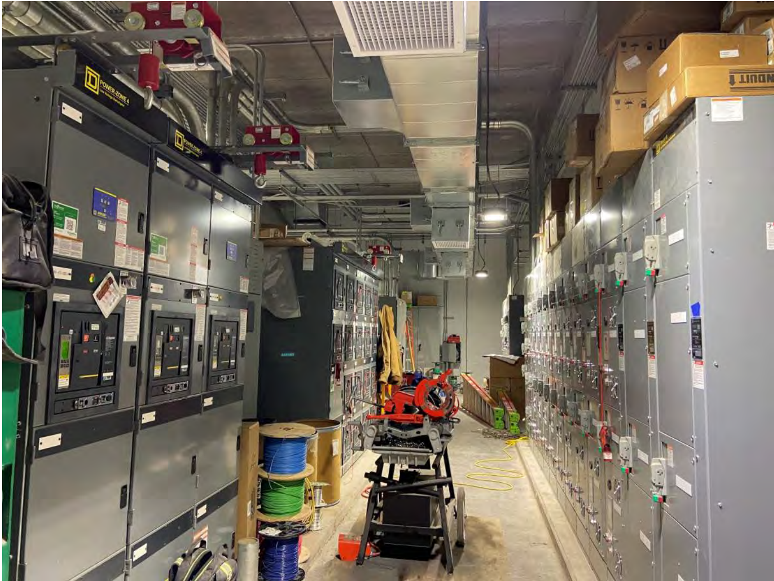
Electrical Room – Much of the equipment is operational
