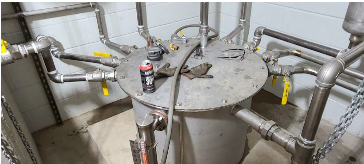
New Digester Gas accumulator, piped up and ready for action
