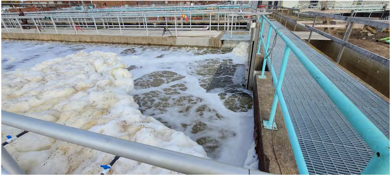
Blower and diffusers at Structure 410 (Activated Sludge Basins) running on full basin to check system out.
