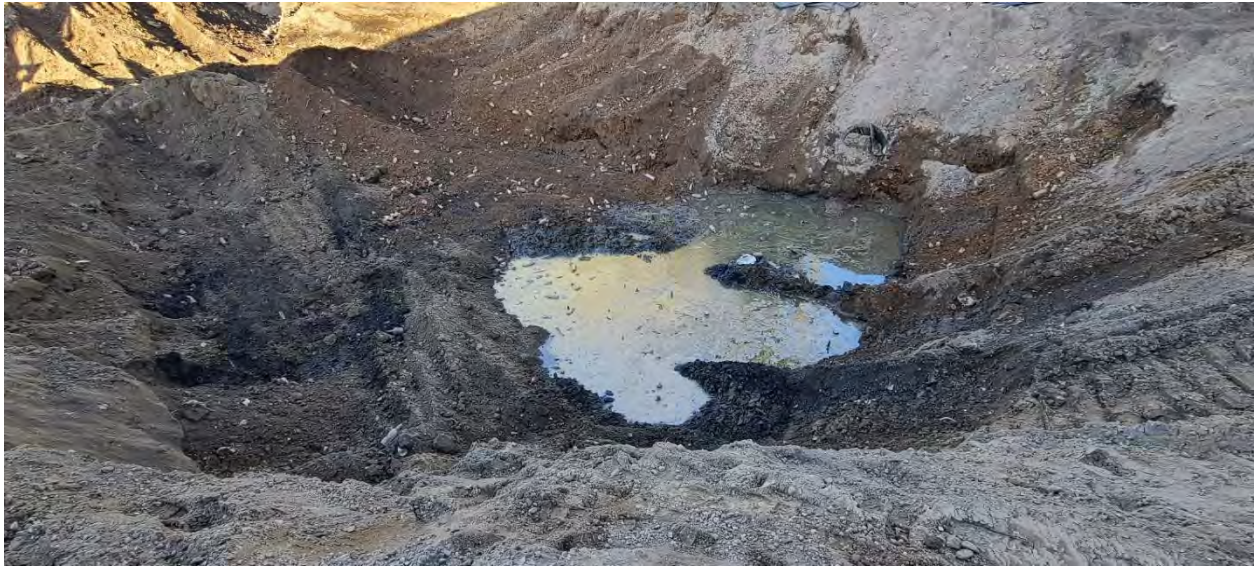
Poor subgrade material for the base layer of the storm water detention system.
