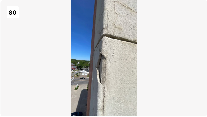
North elevation along the west side of the column concrete delamination reference note for
