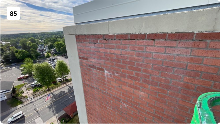
Repair roof concrete coping on North elevation Eastside up to eight linear feet sea reference note 14
