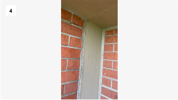
Southwest elevation interior column, caulking at perimeter and two verticals along grid line E to D and 4
