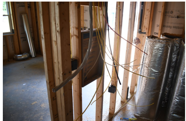
Photo 16 Unit A Mech
