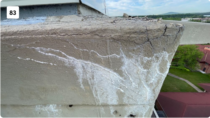
West exterior Corner coping disintegration undercoating reference note 14
